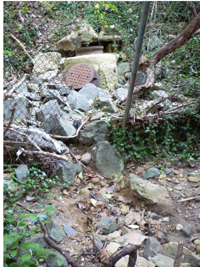
2.20 The manhole cover marking the connection between a 36-inch stormwater line and the 21-inch combined sewer line, September 2013. The cover is repeatedly ejected through the fence and into the park during combined sewer overflows.
