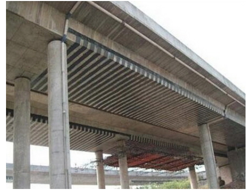
(b) Carbon-fiber composite application to a bridge repair (photo courtesy of StablWall [9]).
