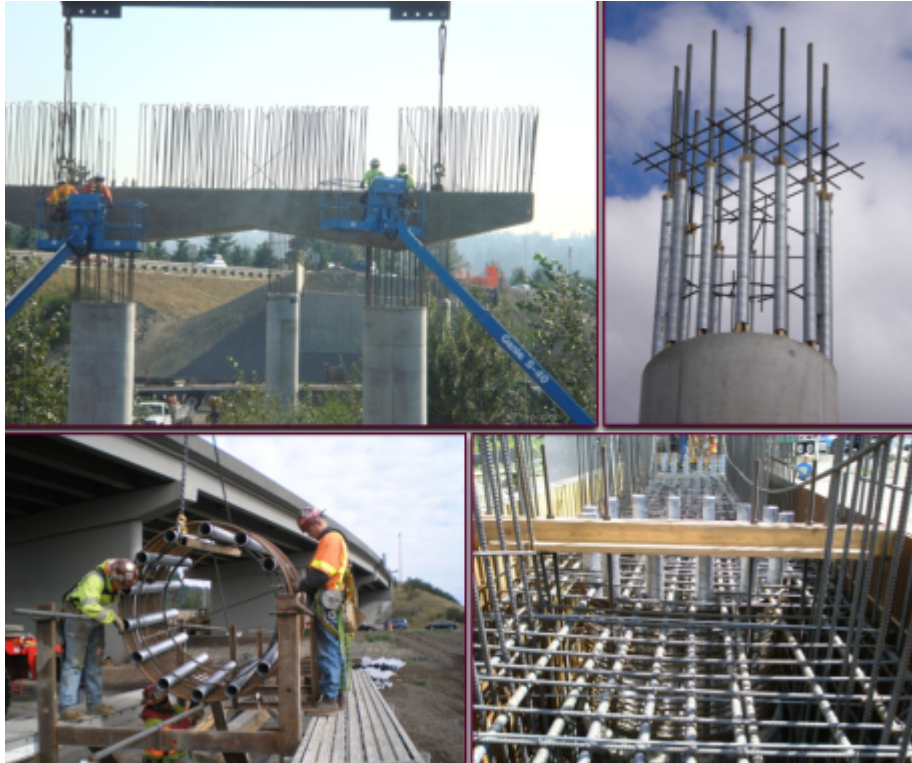
Figure 1.2: Precast Bent Cap Construction in the State of Washington (Marsh et al., 2013)
