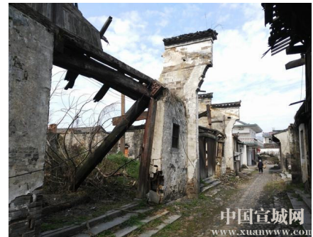
Figure 4. Building collapse due to no maintenance, Zhangdu historical village, Anhui
