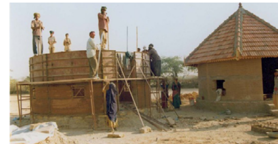
Figure 66: Community work, 2011 @ Hunnarshala. Figure 65-66: In 2001, after the earthquake in Bhuj, Abhiyan, Hunnarshala provided technical guidelines and manual that enabled more than 100 villages to rebuild using earth technologies.
