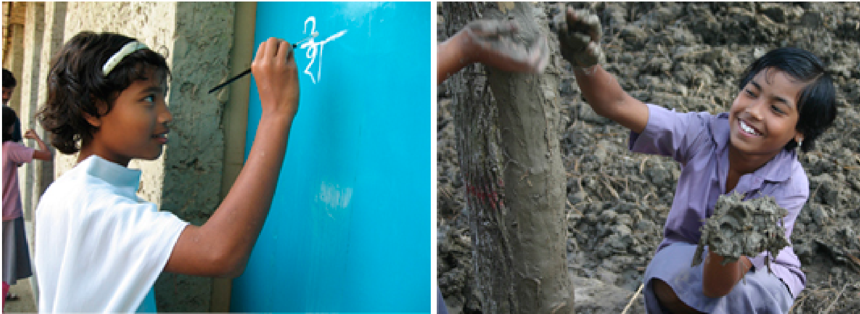
Figure 78: In the afternoon “school construction” was part of the curriculum. The METI students were helping to build their own school - preparing the lintel for example or drying the sand. In the end every student subscribed with the name on the front doors of the school. A yearly expanding school-cronicle. Photos: construction team.
