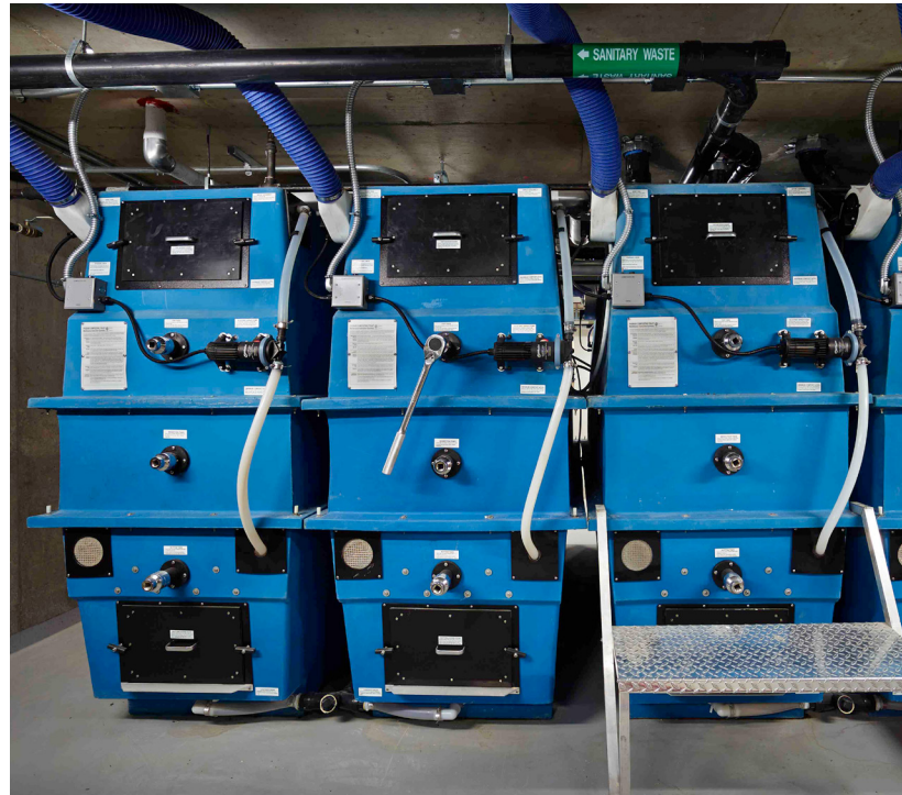
Fig 3.4 Bullitt Center Basement Composters
