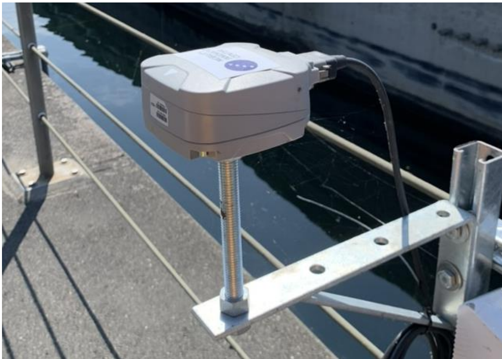
Figure 15. AGM-1 GNSS Receiver Installed at East End of Bridge (Pontoon R)
