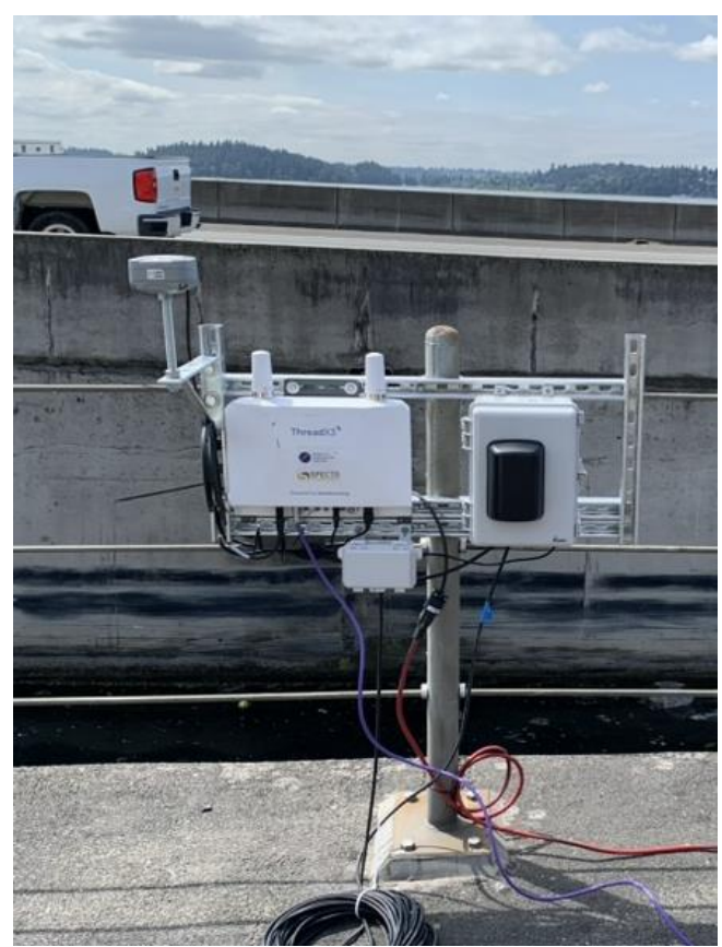
Figure 9. Long-term monitoring setup on eastern end pontoon (Pontoon R)
