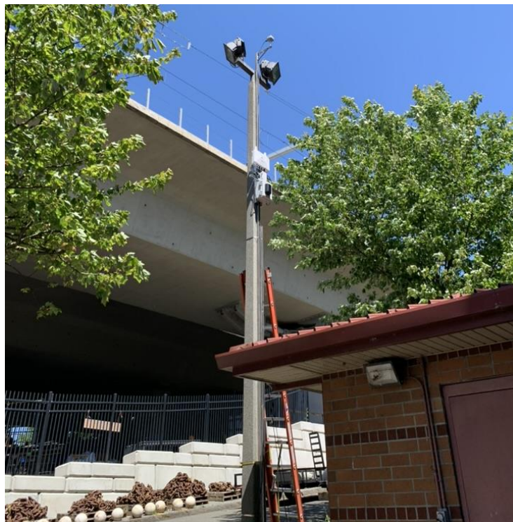
Figure 11. Long-term monitoring base station
