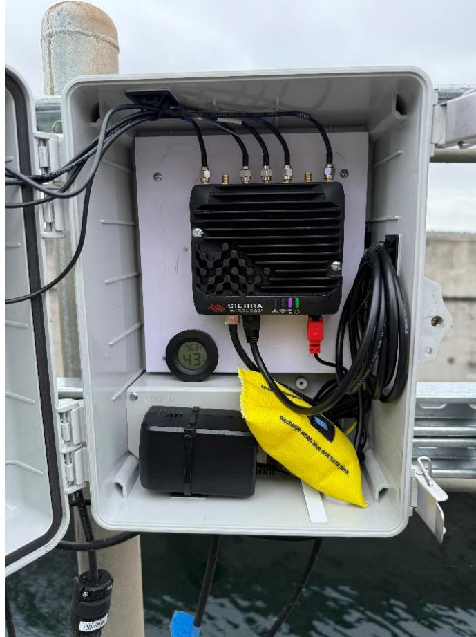
Figure 7. XR60 modem inside enclosure
