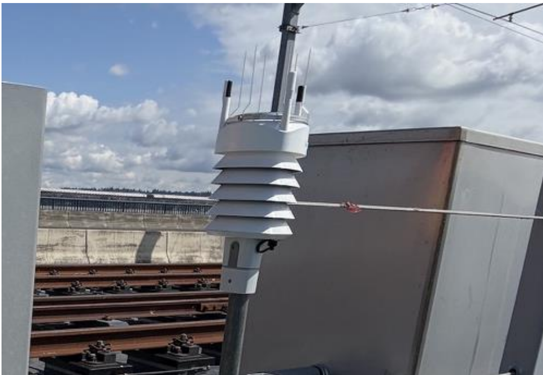
Figure 12. Weather station installed at the midspan of the bridge
