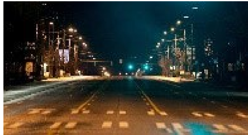
Figure 1-16. Cobra head street lights in Seattle. Photo courtesy of Clearly Sapphire
