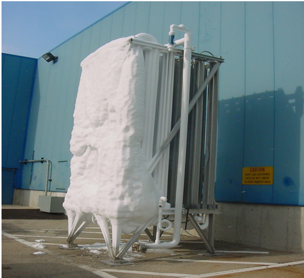
Figure 1.4: An ambient air vaporizer covered in frost. During normal operation frost will begin to develop and continue to grow until either the unit is removed from operation or it suffers catastrophic failure. [7]
