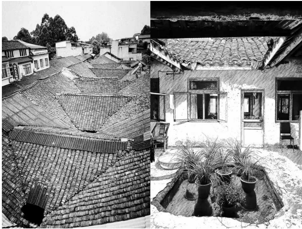
Figure 3.21 A view of “sky wells” for rain water discharge and air exchange in Dantu market
