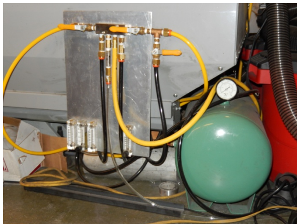
Figure 4.13 Vacuum source control panel
