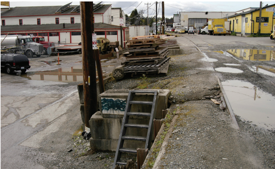
Figure 36. Six foot grade change between the waterfront businesses and NW 54th St
