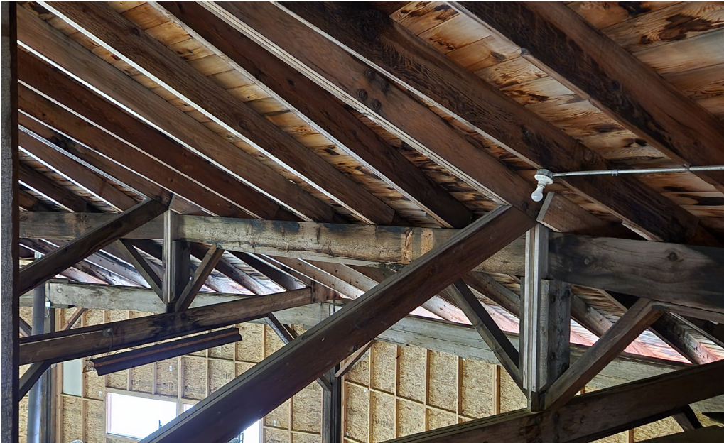
Figure 7: Round House, water damage along roof joists [Image source: Author, Jan. 2023]
