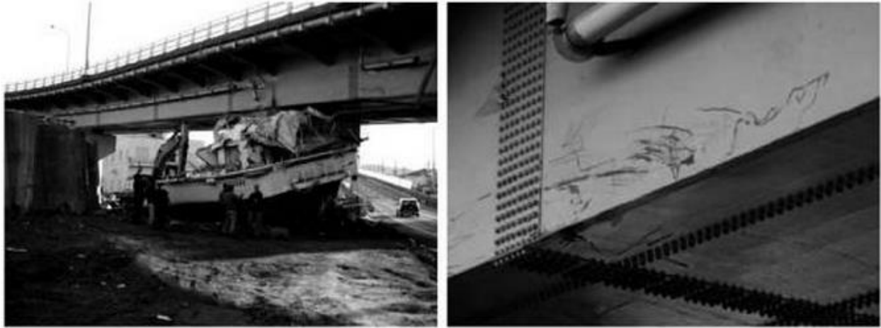
Figure 1-7: Fishing Boat Trapped Below Steel-Box-Girder Bridge (left) (Kriebel), Causing only Superficial Damage (right) (Robertson) (with permission from ASCE)
