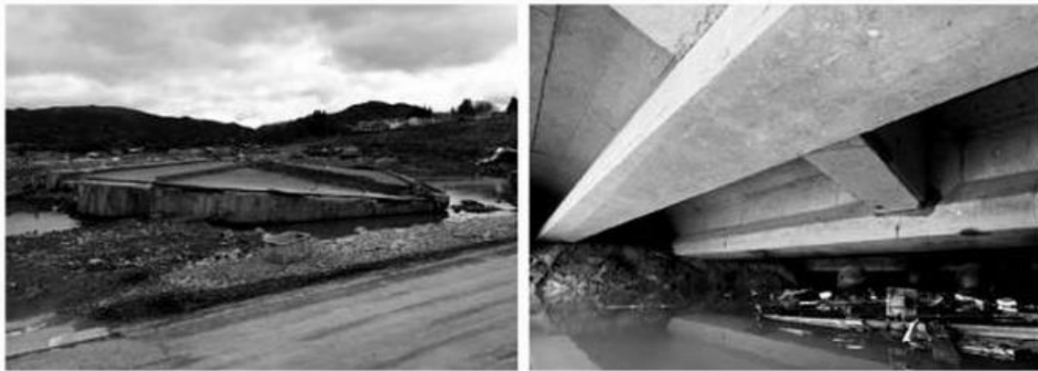
Figure 1-3: Deck Section Displaced from Original Location due to the Uplift (2011 Great East Japanese Earthquake and Tōhoku Tsunami, Robertson, with permission from ASCE)
