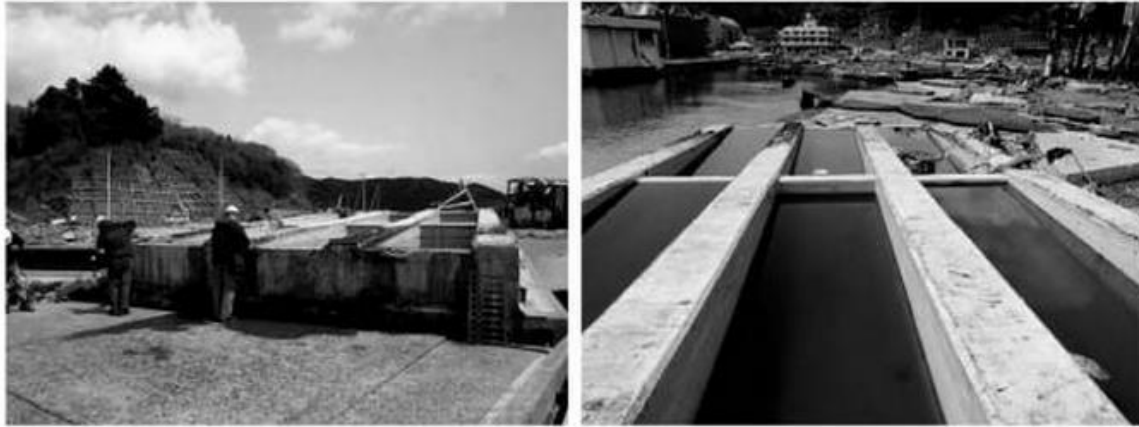
Figure 1-5: Flipped Bridge Superstructures due to the 2011 Great East Japanese Earthquake and Tōhoku Tsunami (Chock (left) & Robertson (right), with permission from ASCE)
