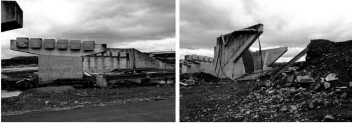
Figure 1-2: Deck Sections Displaced from the Piers and Abutments (left); Severe Scour behind Abutment (right) (2011 Great East Japanese Earthquake and Tōhoku Tsunami, Robertson, with permission from ASCE)
