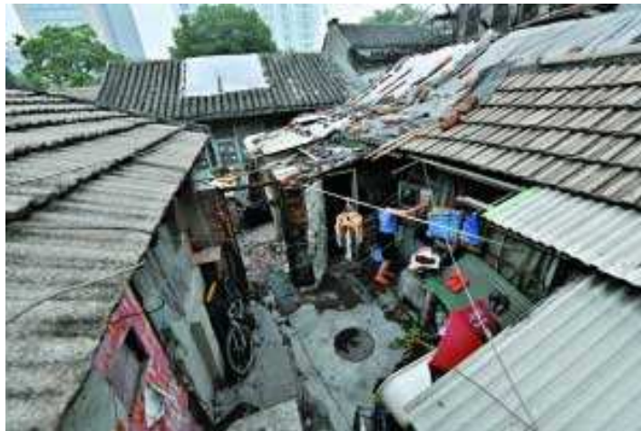
Figure 4.3 A typical dilapidated courtyard house 69
