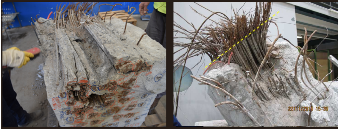
Figure 6.5: Post-collapse observations: (Left) presence of large interior void; (Right) discovery of missing tendon sleeves near the antenna, from [Rosati et al. (2018)]
