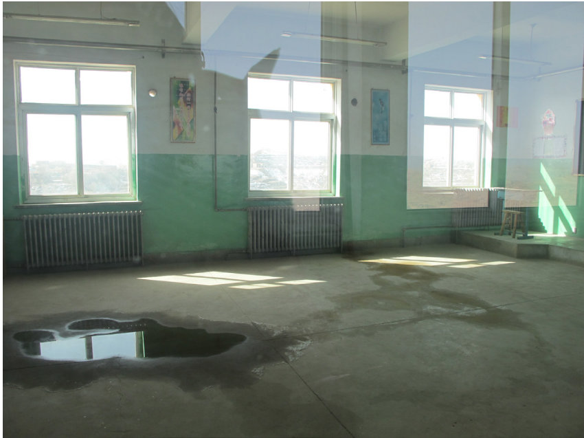
Climate damaged the building construction.
