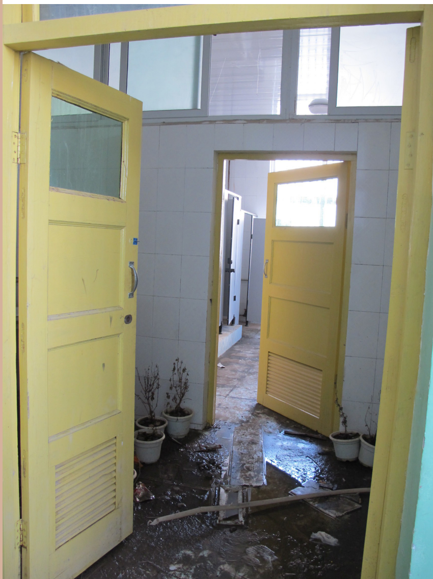
The toilet doesn't work because the pipes cracked due to the coldness.
