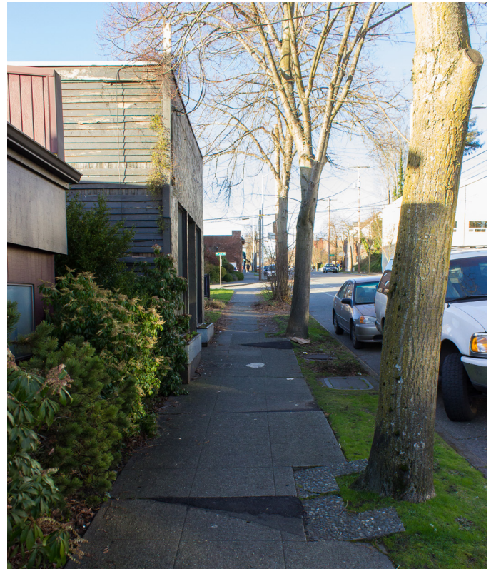
Fig. 4-21: Roosevelt Way NE, facing north from NE 70th St. Current sidewalks along the corridor are barely 6' wide, and many are in substantial disrepair. While there is little room for widening them, many sections need to be repaved to ensure safety and accessibility.
