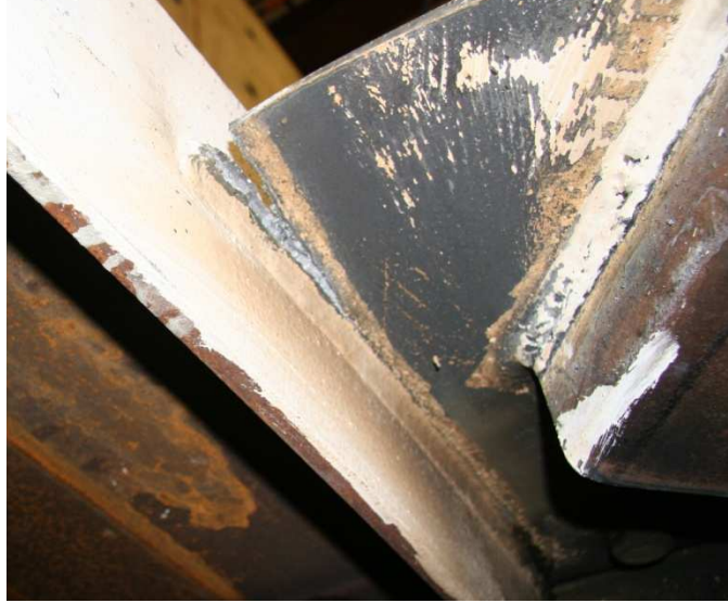
Figure 5.242 W3 in South Gusset-to-Beam Weld
