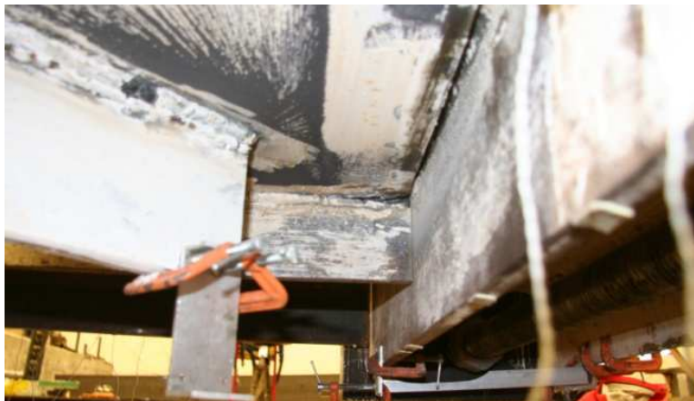
Figure 5.172 W2 in North Gusset-to-Beam Weld
