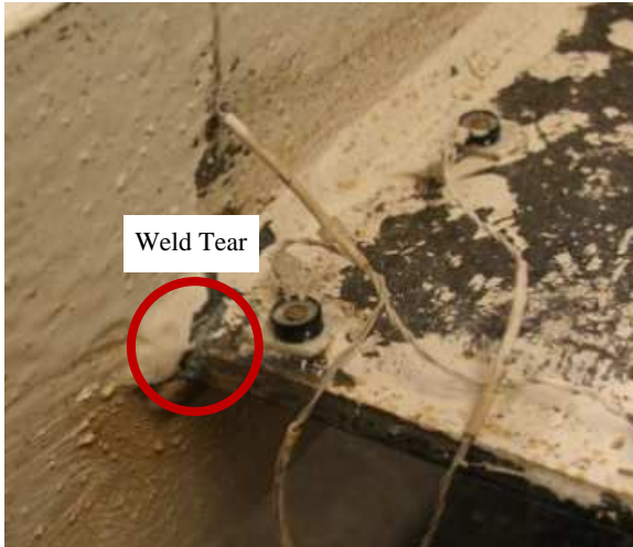
Figure 5.199 W1 in North Gusset-to-Beam Weld
