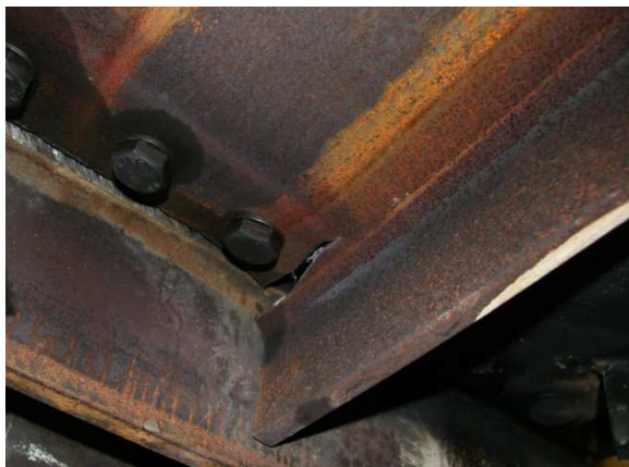
Figure 5.243 Tear in North Beam Web - MT
