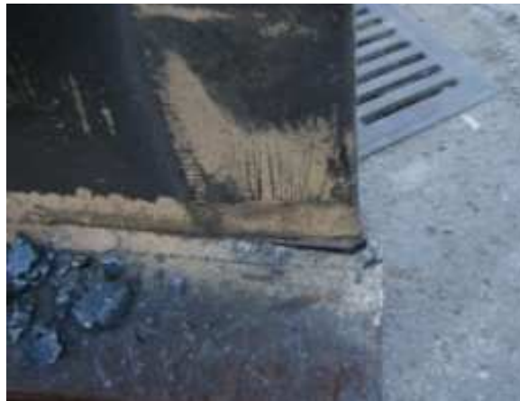
Figure 5.86 W1 in North Gusset-to-Beam Weld (After Disassembly)
