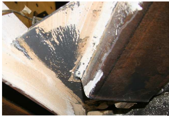
Figure 5.231 Tearing of South Gusset-to-Beam Weld
