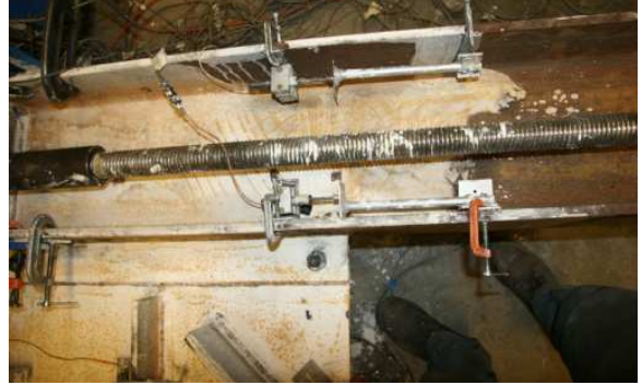
Figure 5.144 Existing Damage to West Column Web
