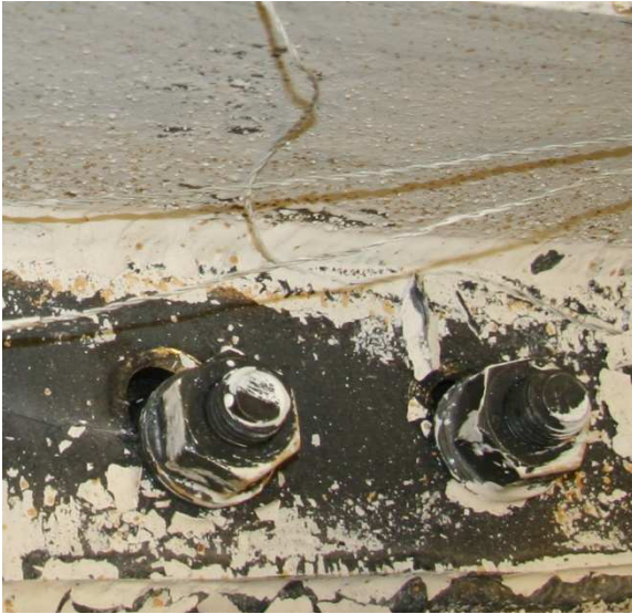
Figure 5.23 Bolt Hole Elongation - BTE NCBF1-R5
