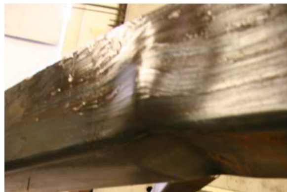
Figure 5.38 Brace Cupping - BC
