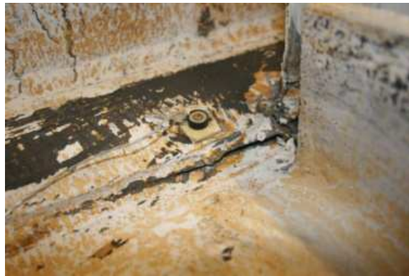
Figure 5.122 North Beam-to-Shear Tab Weld - W2 and North Shear Tab - MT
