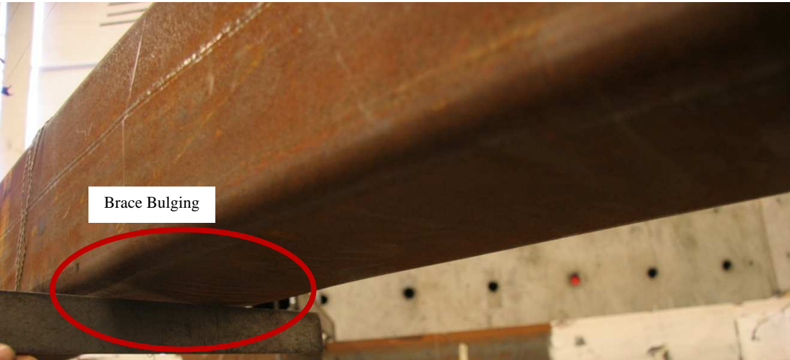
Figure 5.191 Bulge 3.5" SW of Brace Center
