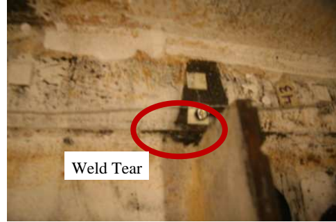
Figure 5.80 New Tear in North Beam-to-Shear Tab Weld
