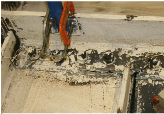
Figure 5.230 Tearing of North Beam-to-Shear Tab Weld
