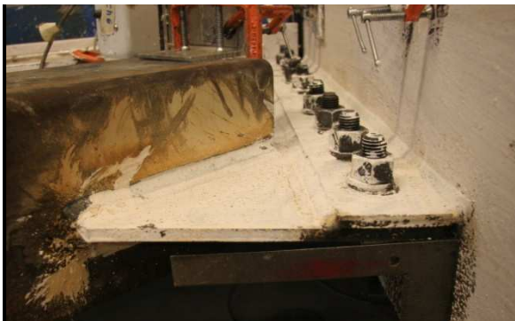
Figure 5.187 Upward Bending of South Gusset Plate
