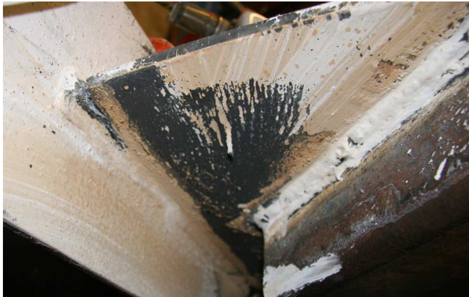
Figure 5.224 W2 in South Gusset-to-Beam Weld
