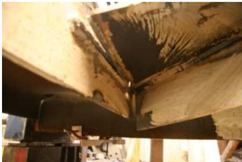
Figure 5.129 Increased Tearing in North Gusset-to-Beam Weld
