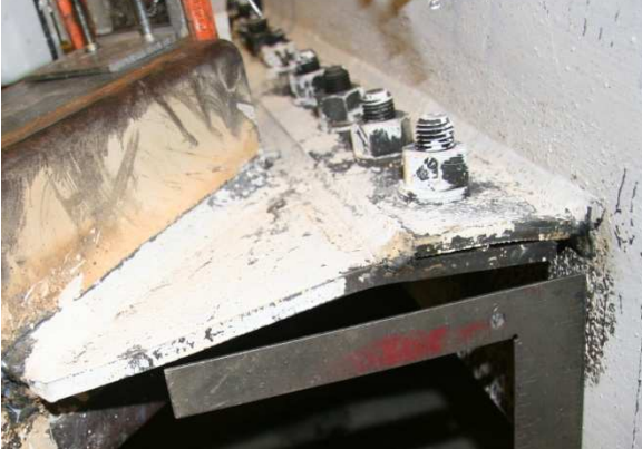
Figure 5.227 Bending of South Gusset- North
