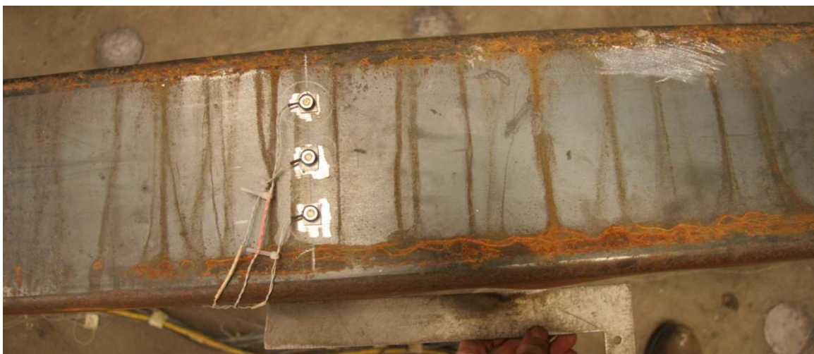
Figure 5.197 Inward Cupping of Brace North Wall
