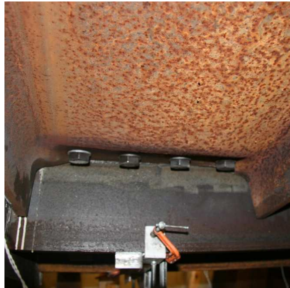
Figure 5.219 Bending of North Beam Web
