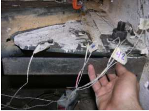
Figure 5.62 North Gusset Plate Bending
