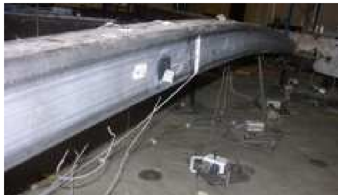
Figure 5.67 Brace Buckling - B2
