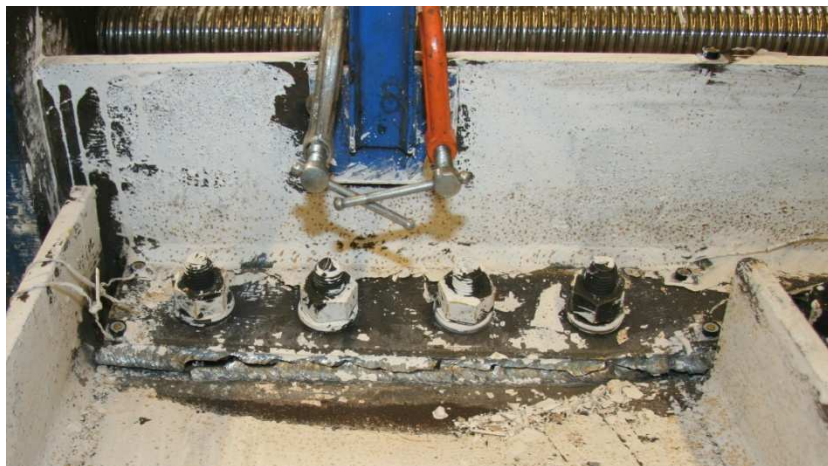
Figure 5.247 Fracture of North Beam-to-Shear Tab Weld
