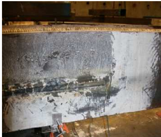
Figure 5.145 Existing Damage to East Column East Flange
