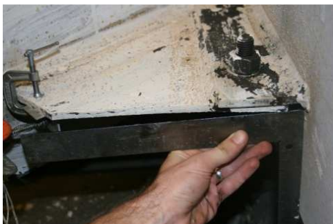
Figure 5.110 Upward Bending of N Gusset Plate
