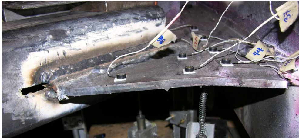
Figure 5.52 Downward Hinging of South Gusset Plate
