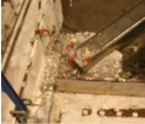
Figure 5.87 North Gusset Plate - Y3
