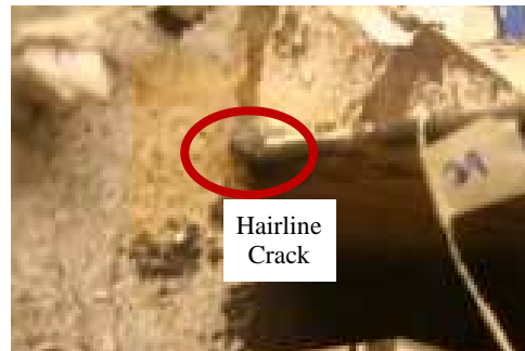
Figure 5.77 W1 in North Gusset-to-Beam Weld
