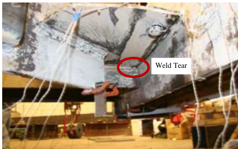
Figure 5.164 W1 in North Gusset-to-Beam Weld
