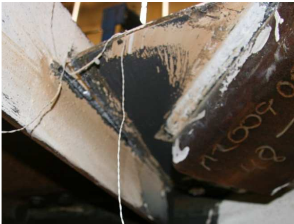
Figure 5.211 WF in North Gusset-to-Beam Weld
