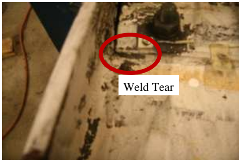
Figure 5.76 W1 in North Beam-to-Shear Tab Weld
