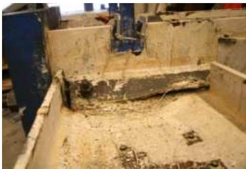
Figure 5.132 W3 in North Beam-to-Shear Tab Weld
