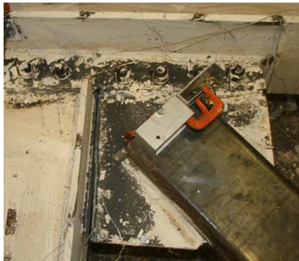
Figure 5.22 Weld Fracture - WF NCBF1-R5
