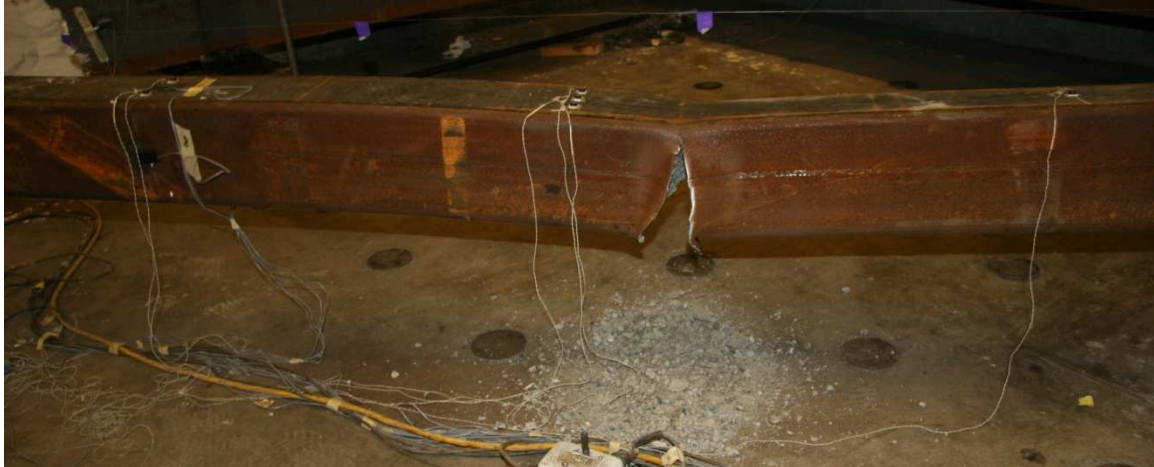
Figure 5.232 Tearing of Brace
