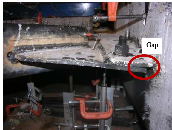
Figure 5.70 Bending of South Gusset Plate from Shear Tab
