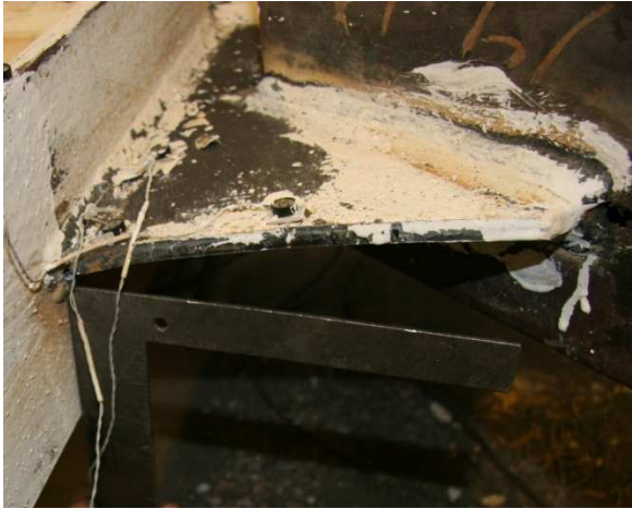
Figure 5.206 North Gusset Plate Bending
