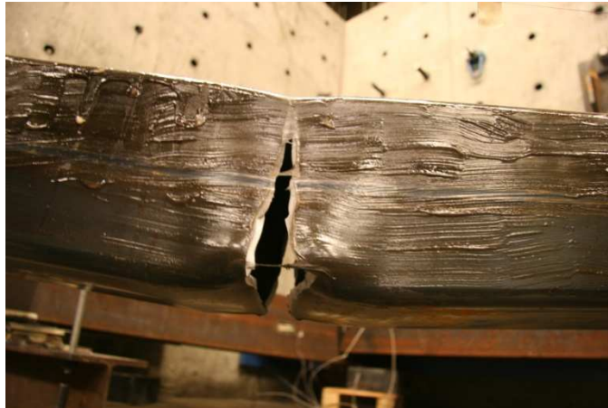
Figure 5.41 Mid-Cycle Brace Tearing
