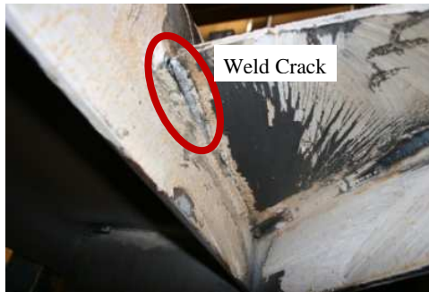
Figure 5.123 W3 in North Gusset-to-Beam Weld
