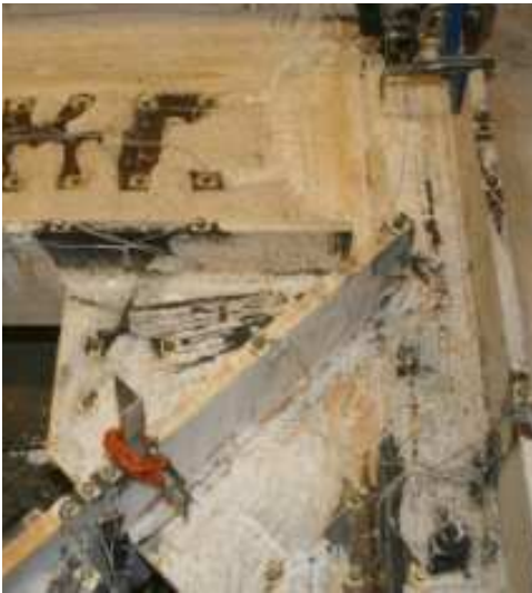
Figure 5.102 North Gusset Plate - Y2
