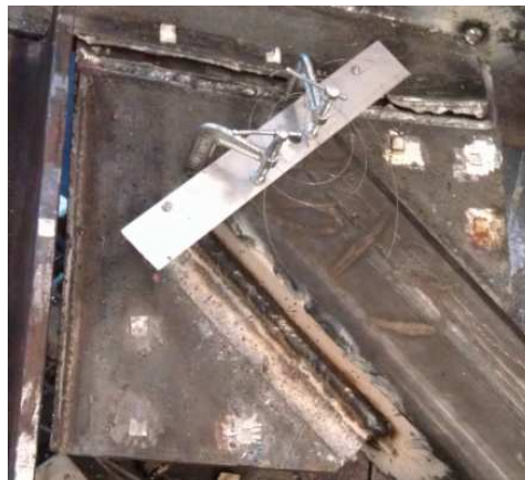
Figure 5.55 Fracture of North Gusset-to-Beam and Gusset-to-Shear Tab Welds
