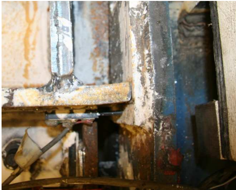
Figure 5.16 Column Flange Buckling - LB NCBF1-R3
