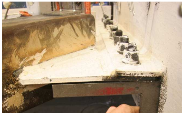
Figure 5.188 Downward Bending of South Gusset Plate
