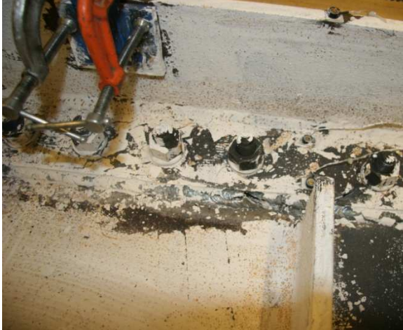
Figure 5.220 W3 in North Beam-to-Shear Tab Weld
