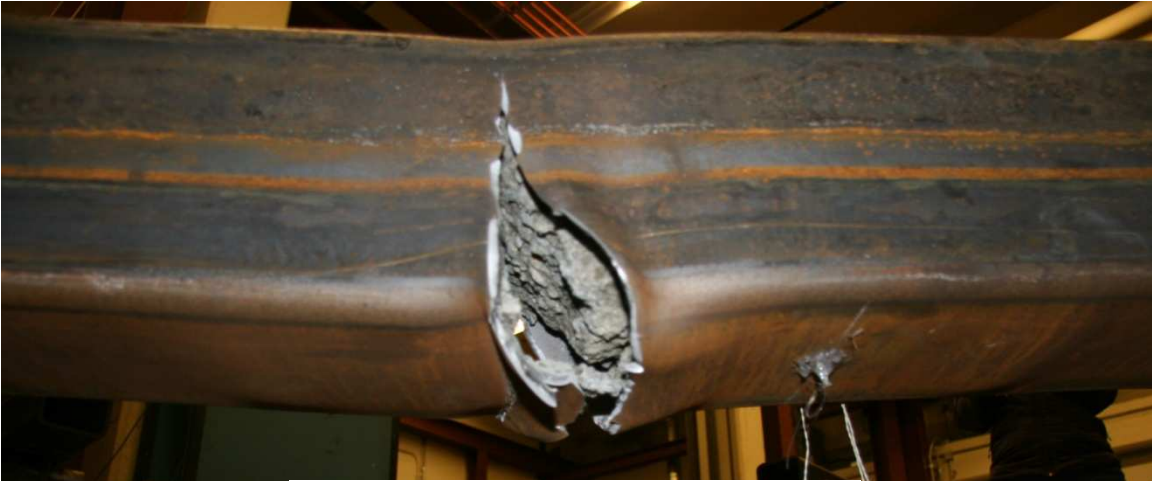
Figure 5.225 Tearing of Brace
