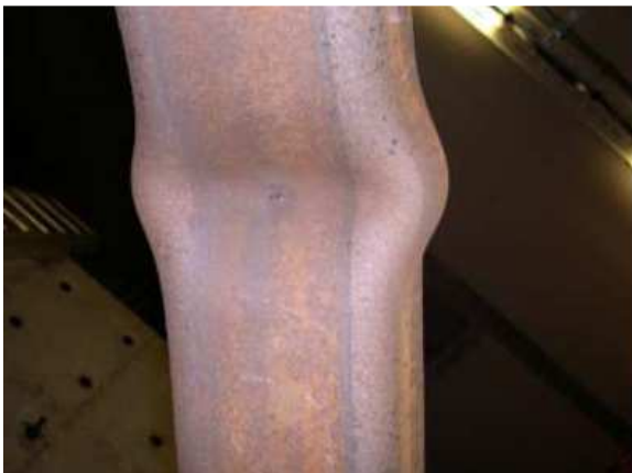
Figure 2.6 HSS18 Brace Cupping (Powell 2010)
