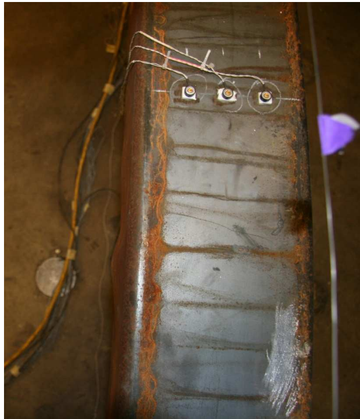
Figure 5.204 Bulges in Brace North Wall
