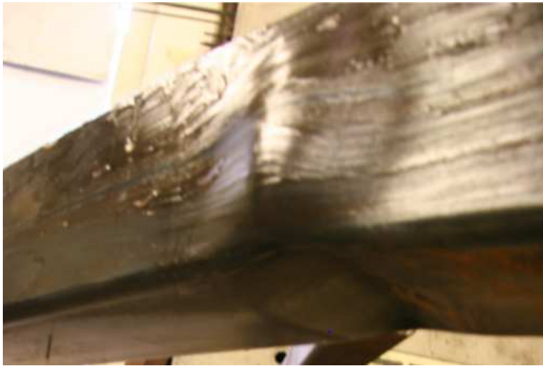
Figure 5.12 Brace Cupping - BC NCBF1
