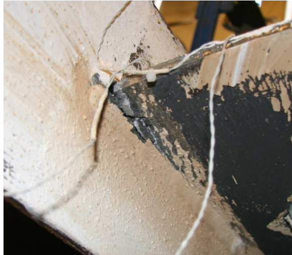
Figure 5.20 Moderate Weld Tearing - W2 NCBF1-R5
