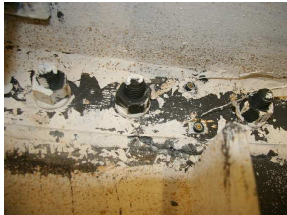
Figure 5.212 Weld Crack W-NBS - W2
