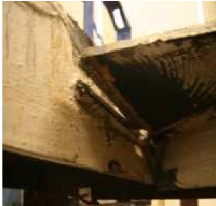
Figure 5.131 Fracture of North Gusset-to-Beam Weld
