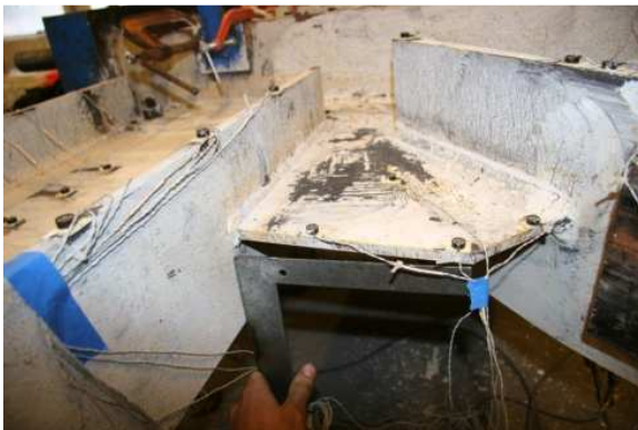
Figure 5.161 North Gusset Plate Bending
