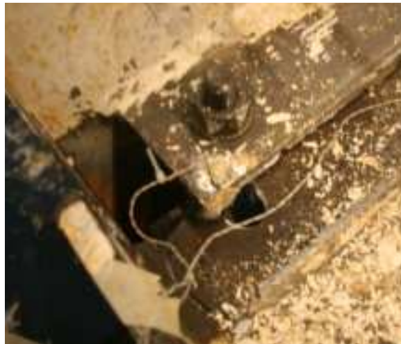
Figure 5.138 Erection Bolt Pullout from North Beam Web
