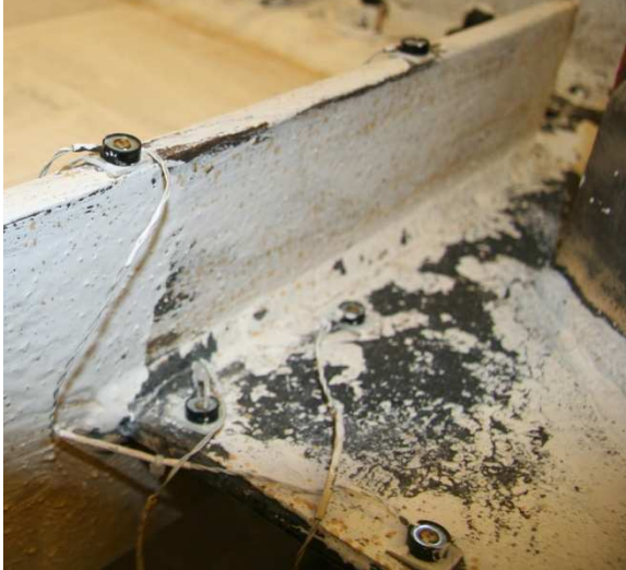
Figure 5.19 Initial Weld Tearing - W1 NCBF1-R5
