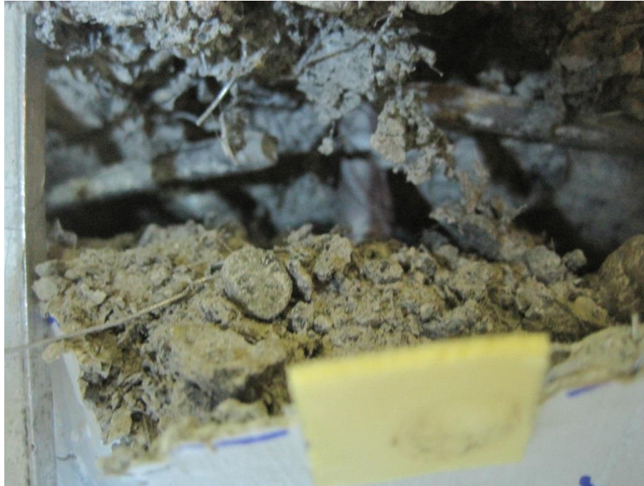
Figure C - 12: Fracture of longitudinal reinforcement bar, cycle 9-2.
