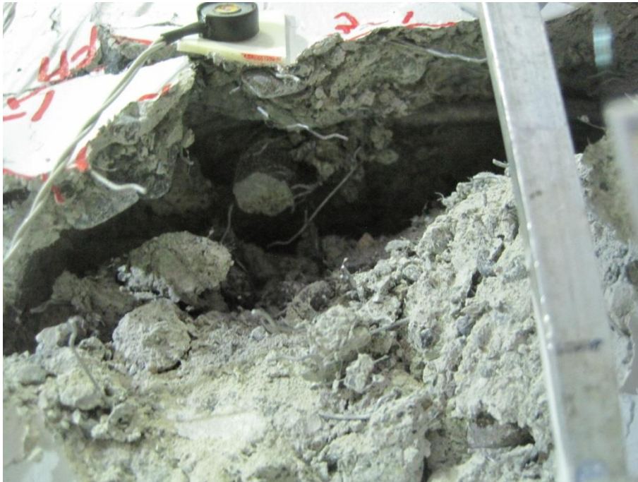
Figure C - 5: Fracture of longitudinal reinforcement, cycle 8-1.
