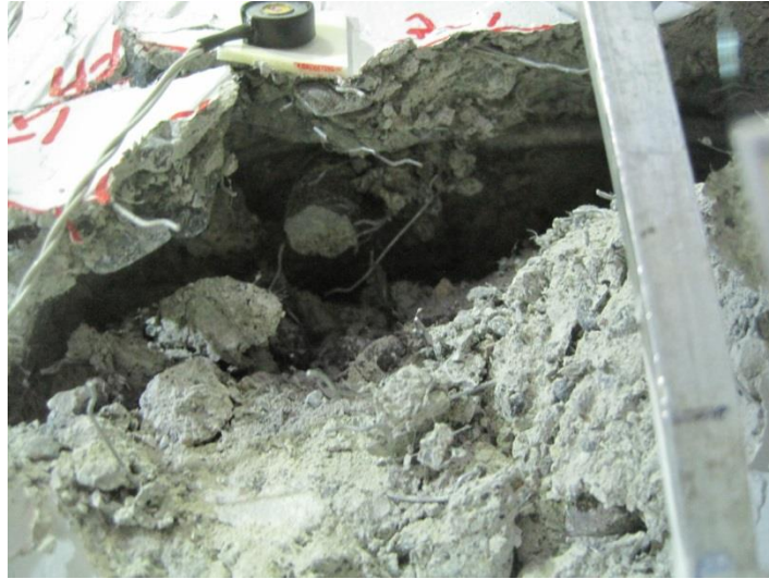
Figure 4-8: PreT-BS broken longitudinal rebar.
