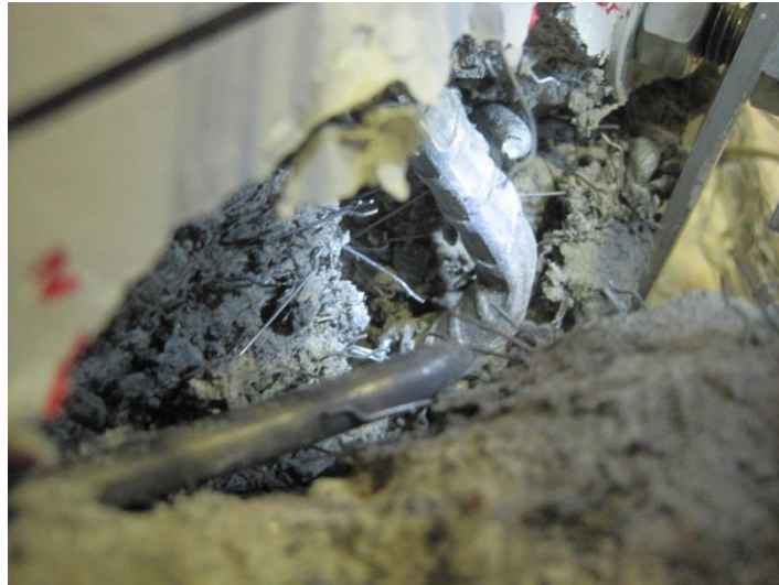
Figure 4-9: PreT-SS buckled rebar and broken spiral.
