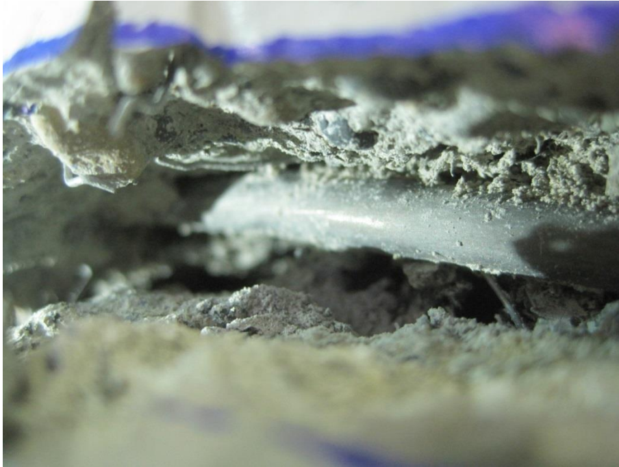
Figure C - 4: Large crack in concrete core, cycle 9-1.
