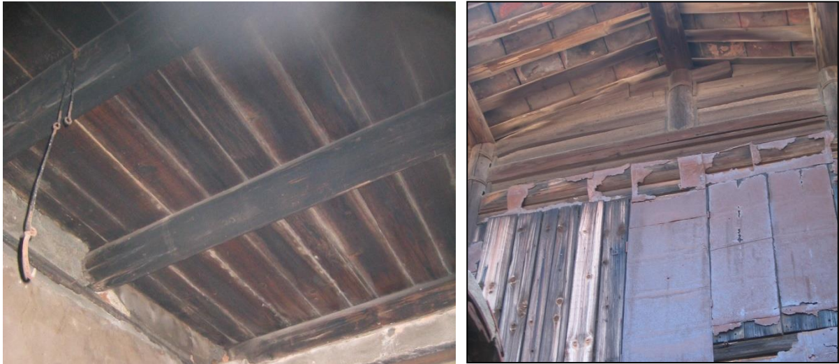
Fig. 35: Photos of aged wood structure in a property (Werkhart International, 2005).
