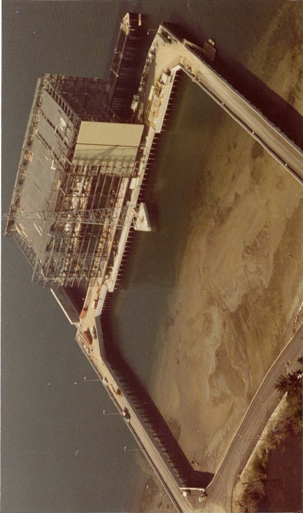
Plate I. The Explosives Handling Wharf (EHW) during construction showing trestles, pilings, submarine berth area (upper right), and partially completed enclosure. Photo taken 2/77, pier completed 2/78.
