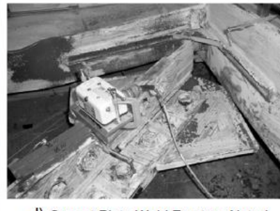
d) Gusset Plate Weld Fracture Noted with BRB06
