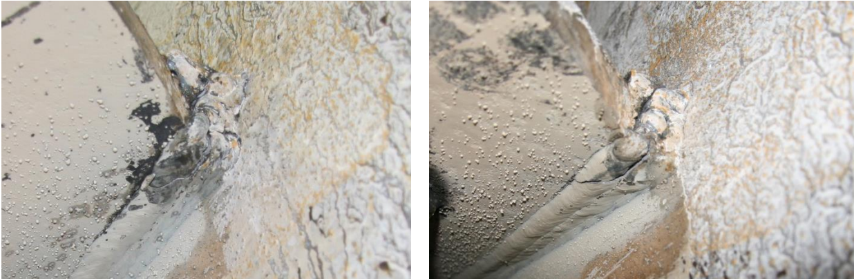
a. SW Gusset Plate - N End of Weld
