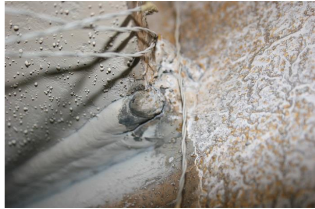
b. NE Gusset Plate – S End of Weld
