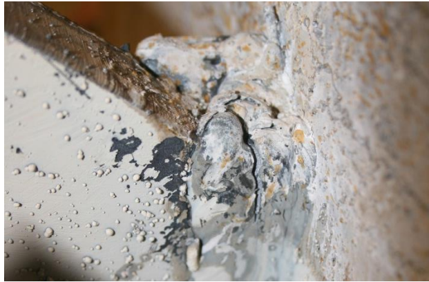
a. SW Gusset Plate - N End of Weld
