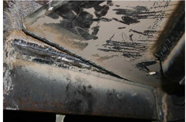
b. NE Beam-to-Gusset Plate Weld Tear at 2.9%
