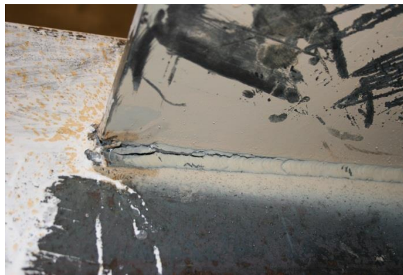
Figure 5-15: Severe Weld Tear in SW Beam-to-Gusset Plate Weld (PS W3, 2.3%)
