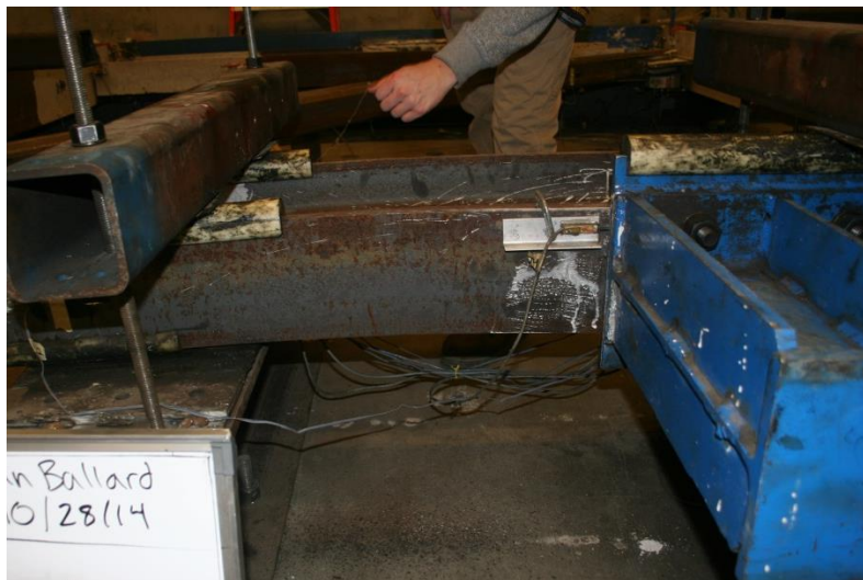
Figure 5-66: Global Buckling of N Beam (2.7%)
