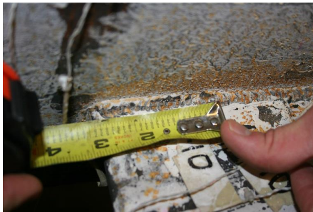
Figure 5-11: Weld Damage in NE Beam-to-Gusset Plate Upper Fillet Weld (1.6%)
