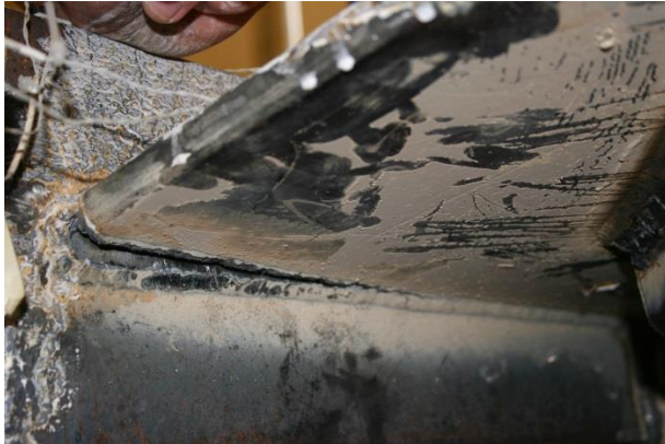
a. NE Beam-to-Gusset Plate Weld Tear at 2.4%
