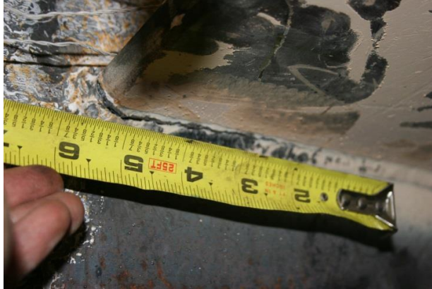
Figure 5-10: Severe Weld Tearing in NE Beam-to-Gusset Plate Weld (PS W3, 1.6%)
