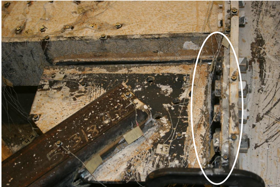
Figure 5-19: NE Gusset Plate-to-End Plate Weld Fracture (PS W4-WF, 2.9%)
