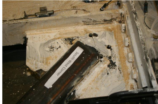
b. SW Corner Gusset Plate Yielding
