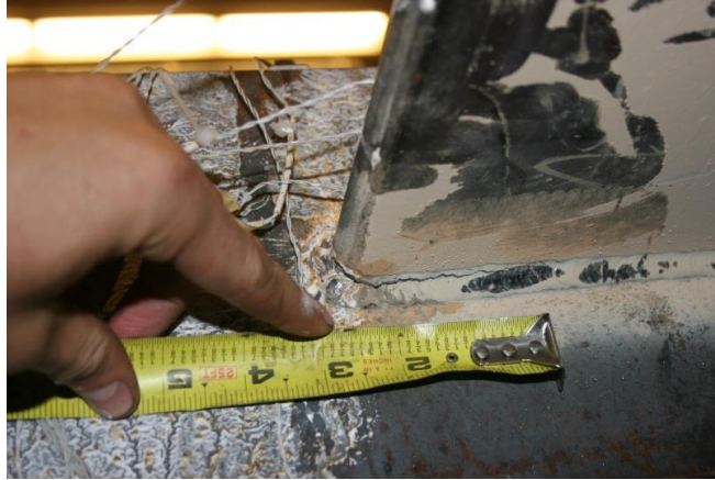
Figure 5-8: Initial Weld Cracking in NE Beam-to-Gusset Plate Weld (PS W1, 1.1 %)
