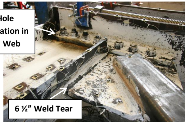
(5) NE Connection Damage at End of Test
