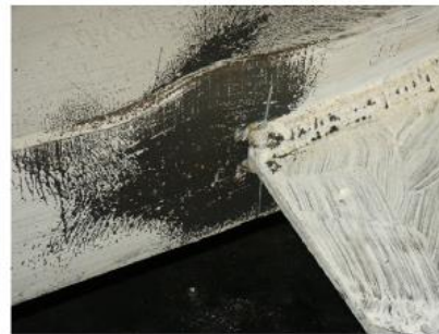
b) Beam Flange Fracture Noted with BRB01
