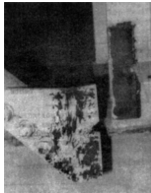
(c) Fractured gusset-plate-to-column weld
