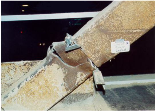
(a) Fractured brace (Kelly et al. 2000)
