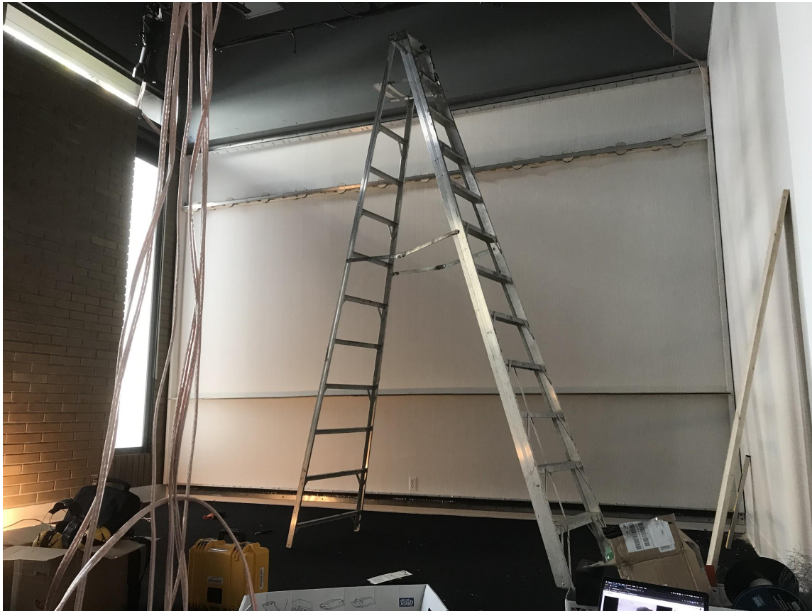
Figure 60 - Running speaker wire through the rafters to the small projection room over the entryway
