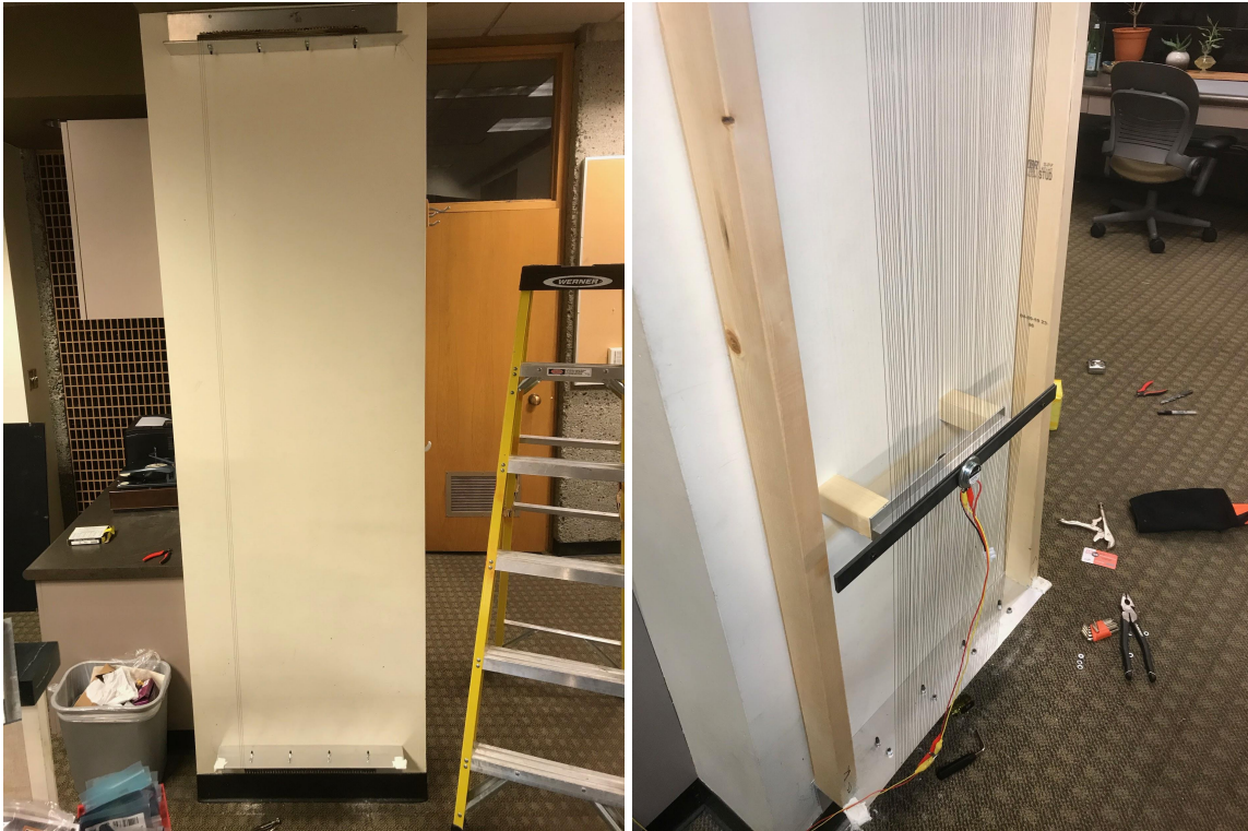
Figure 44 - Seventeen inch wide model of Large String Array
