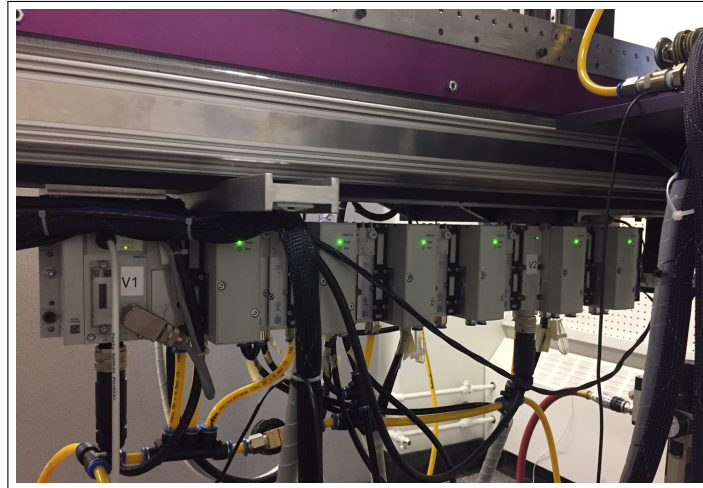
Figure 2.5: Displays the Festo valve manifold utilized to control the pressure outputs to the pneumatic components.
