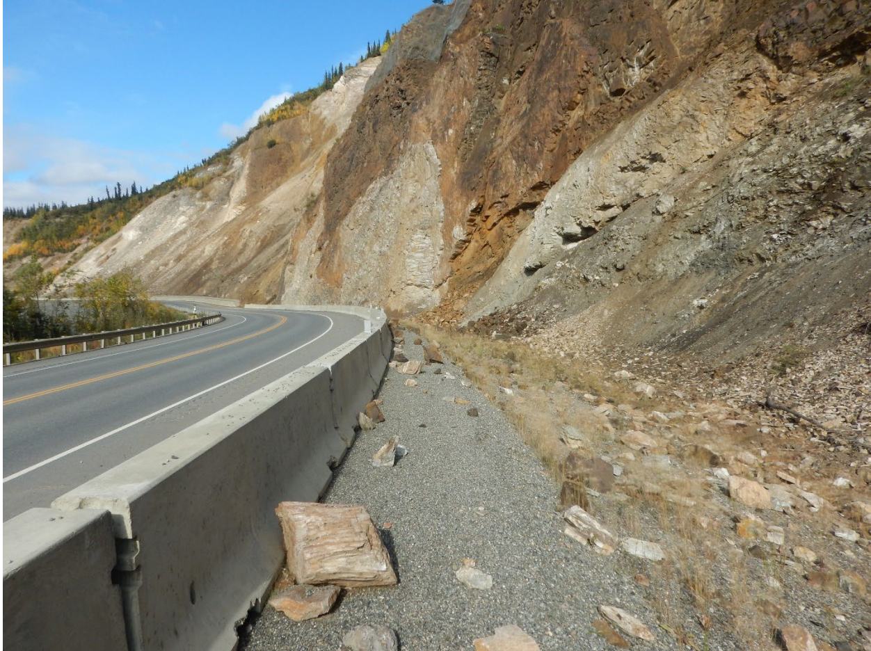
Figure 2.13 Recent rockfall behind barrier along the Parks Highway MP239 rock slope.
