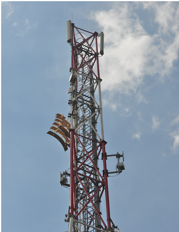
55. Kenya FabFi reflector mounted on existing tower
