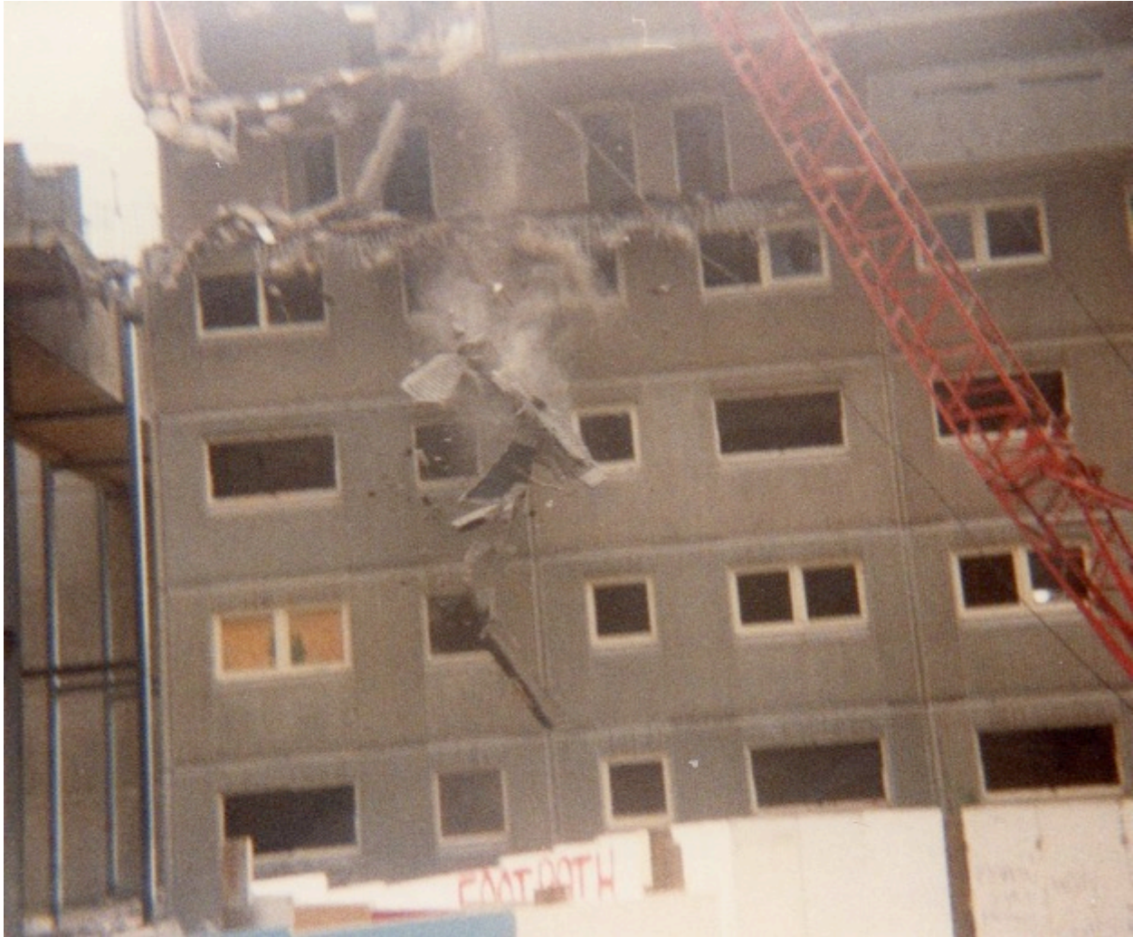
Beginning of the demolition of the Killingworth Towers, 6 August 1987, 3:30 pm. Photo by Dave Gilmore.
