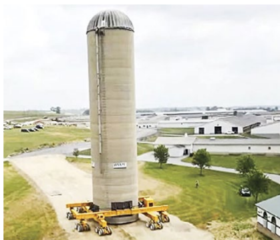
Figure 45: Moving of a silo at Kreider Farms in Manheim, PA to create an observation tower
