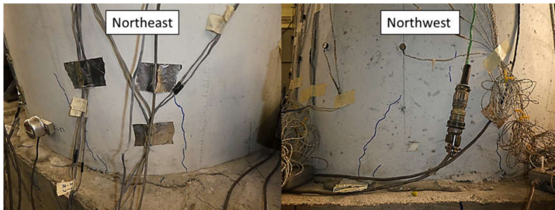
Figure 8-4. Short, fine cracks, Series 2
