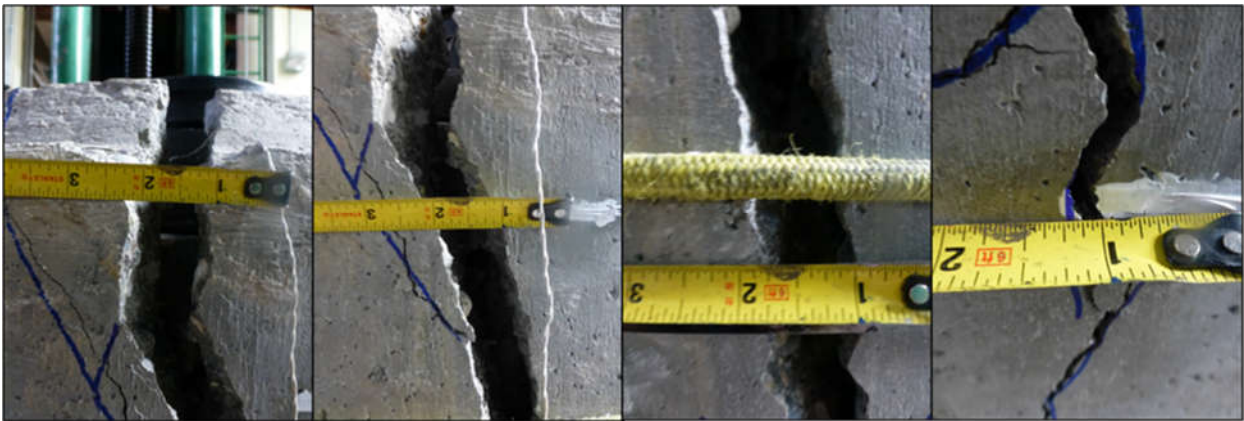
Figure 5-16. Width of large crack on west side of specimen (top to bottom)
