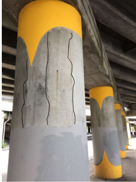
Figure 1-2. Longitudinal cracks on columns of Ravenna Bridge
