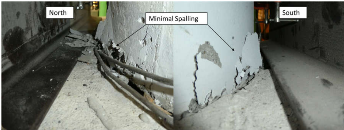
Figure 8-6. Minimal Spalling at base of column, Series 4
