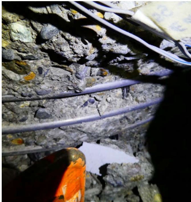
Figure 8-13. Substantial spalling and exposed spiral reinforcement, Series 8
