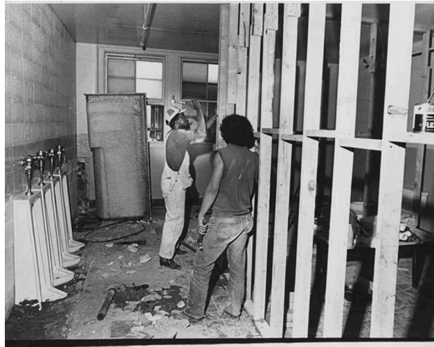
Figure 65: Carpenters Ismael Puente, right, and Thomas Walston working on bathroom in the occupied Beacon Hill School, 1973. (MOHAI 2000.107.124.39.10)
