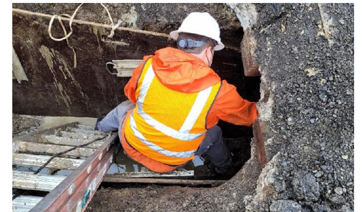
Figure 1: Nick at the bottom of an eight foot hole during construction monitoring, scraping the underside of a historic street car line.
