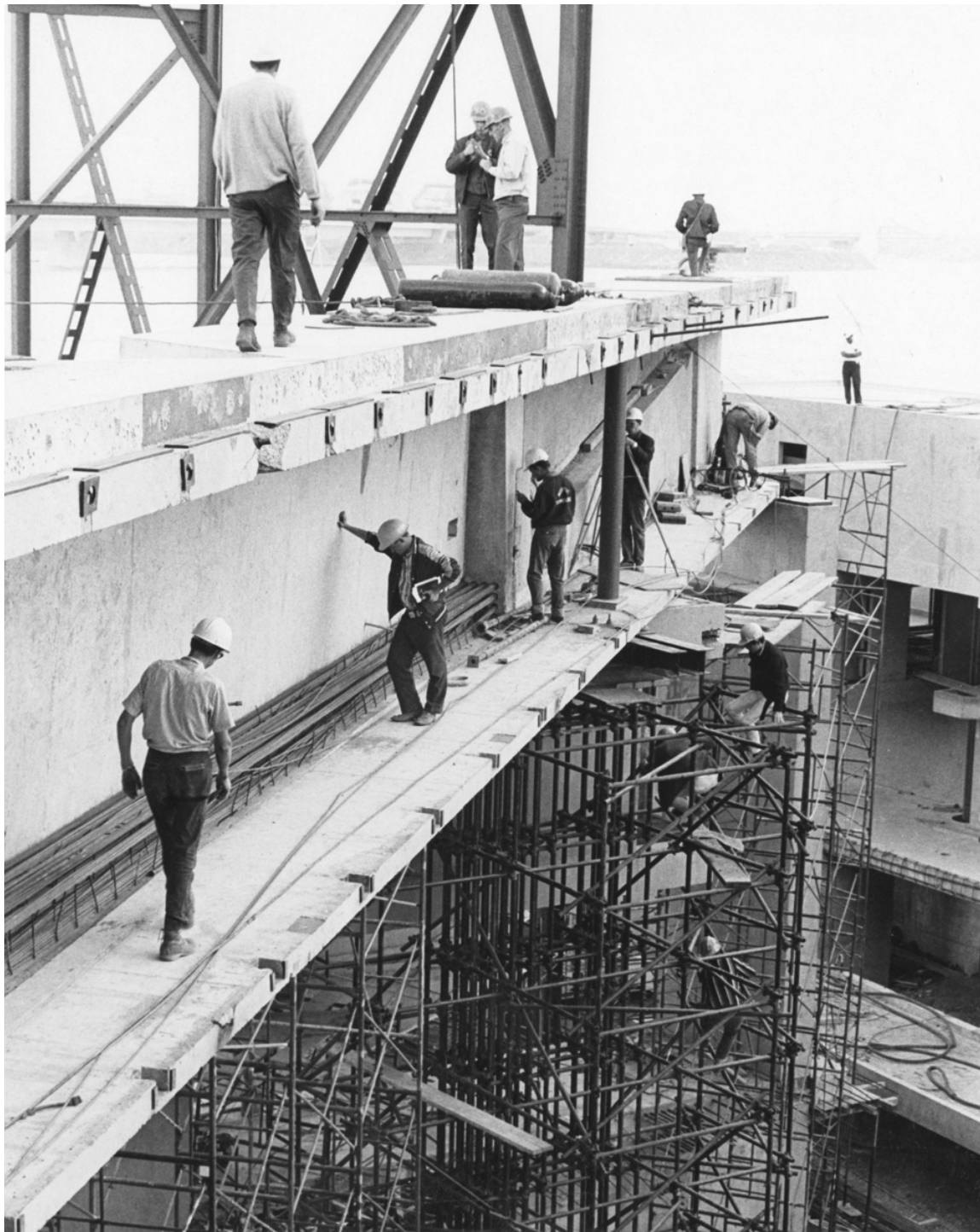
Fig. 54: Construction Site at Habitat 67 1967 Moshe Safdie Archive, Rare Books & Special Collections, McGill University
