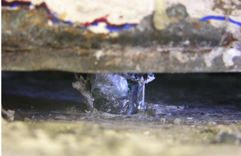
Figure 4.9 Exposed north bar of PreT-SF-ROCK.
