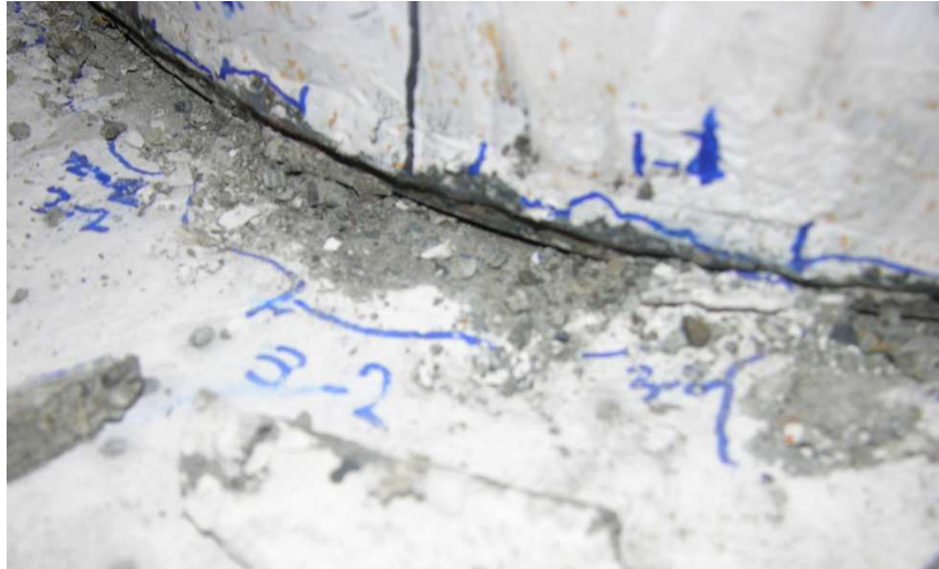
Figure 4.6 South view of PreT-SF-ROCK showing the fillet spalling of the footing induced by the rocking action of the steel shoe.
