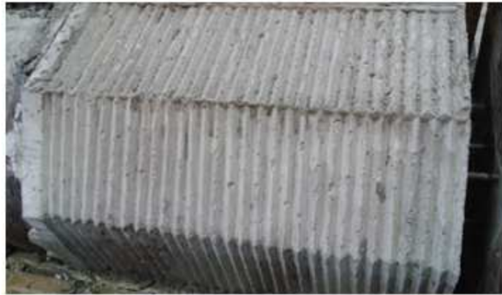
Figure 2.10 Roughened surface of the portion of the column that extends into the spread footing.
