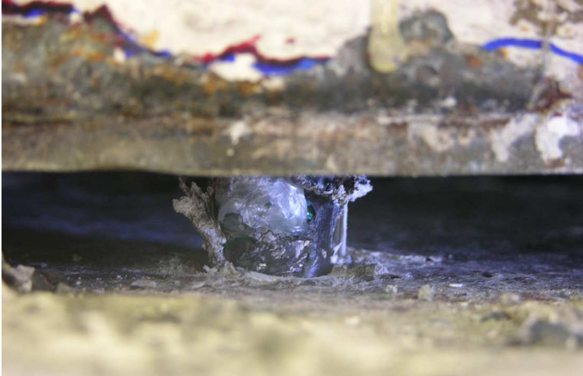
Figure C.11 Exposure of rebar.
