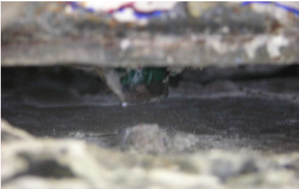
Figure C.12 Fracture of rebar.
