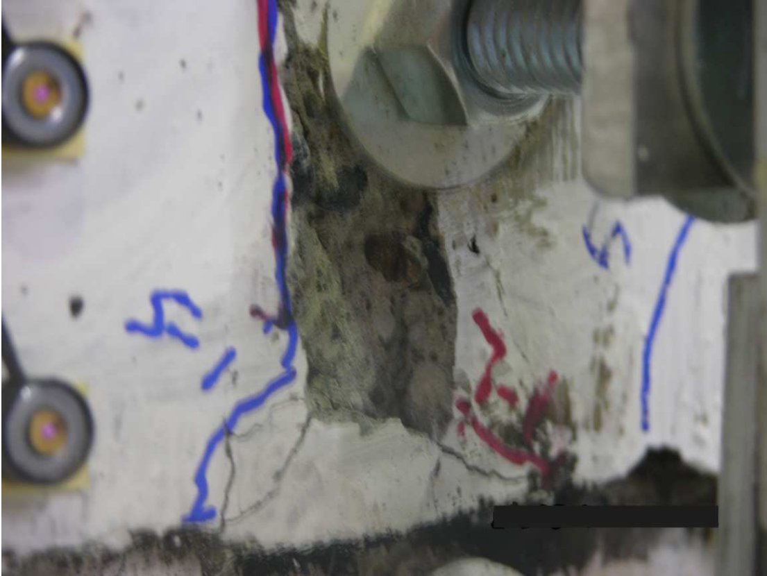
Figure C.9 Cosmetic spalling at top of shoe.
