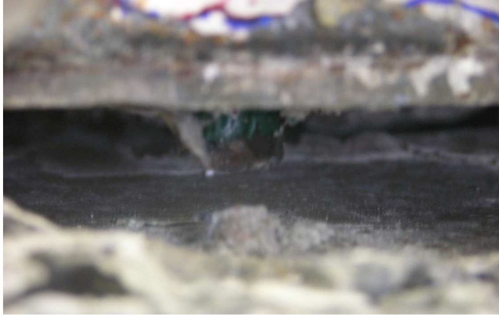
Figure 4.11 Fractured north bar of PreT-SF-ROCK.
