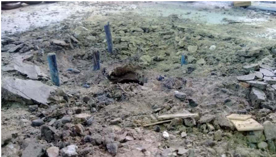
Figure C.7 Top of footing after testing.
