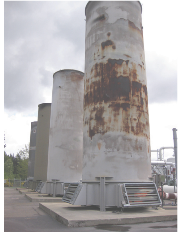
Fig. 4.9 Existing Gas Flares at North end of site.
