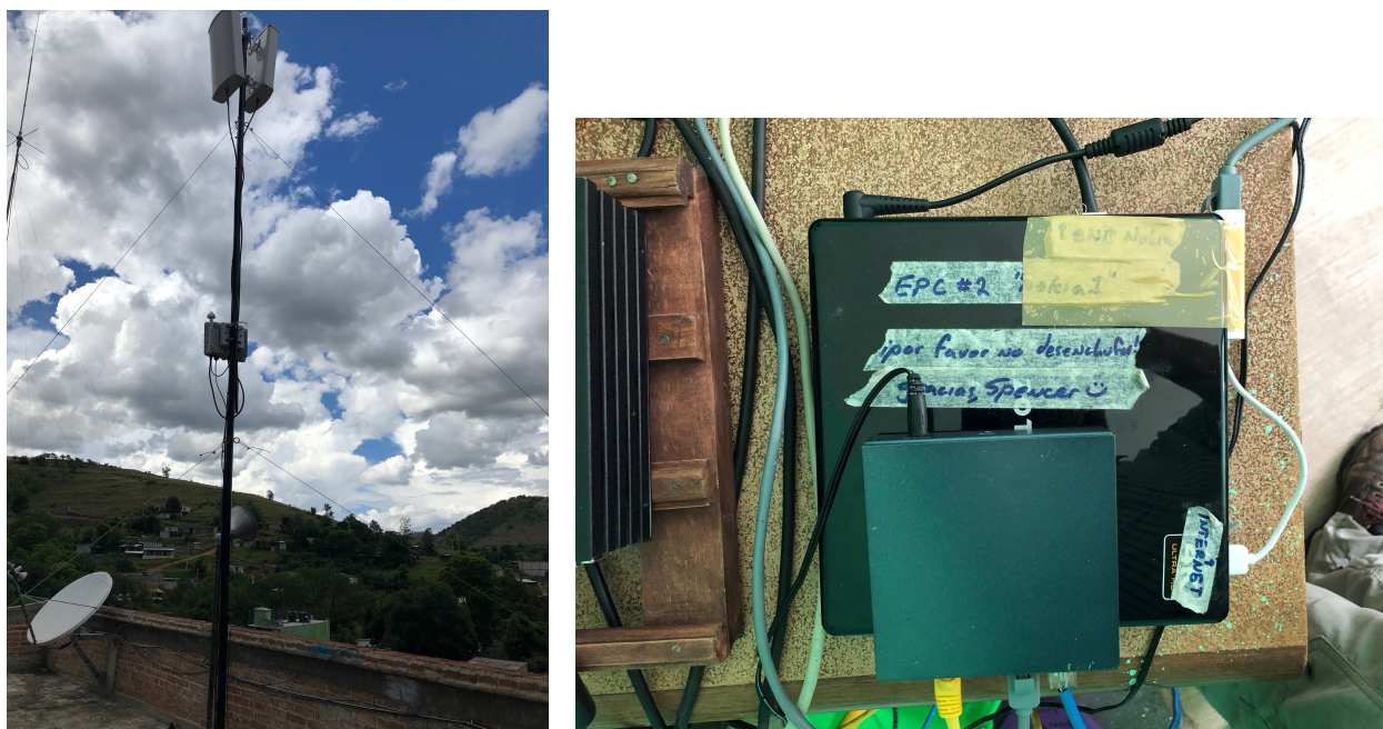
Figure 1.1: Edge CCN hardware. An eNodeB small cell (left) providing coverage over the town center in Santa Inés, and the standalone edge EPC computer (right) serving as the network control and data plane connected to it from the main office. For more information about this network, see Section 6.3
