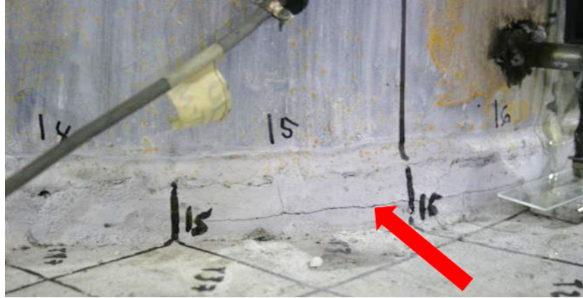
Figure 4.3 Crack below grout pad cusp that resulted from attachment of actuator.
