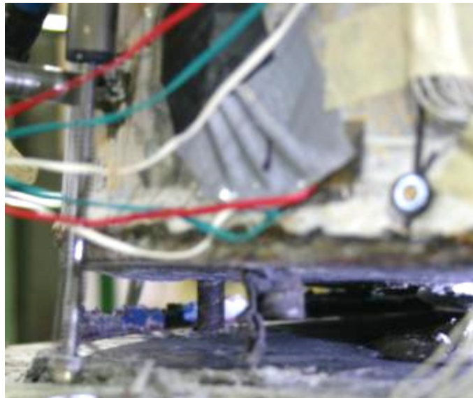
Figure 4.16 Rocking gap after rupture of north most rebar (intact northeast rebar visible in photograph).
