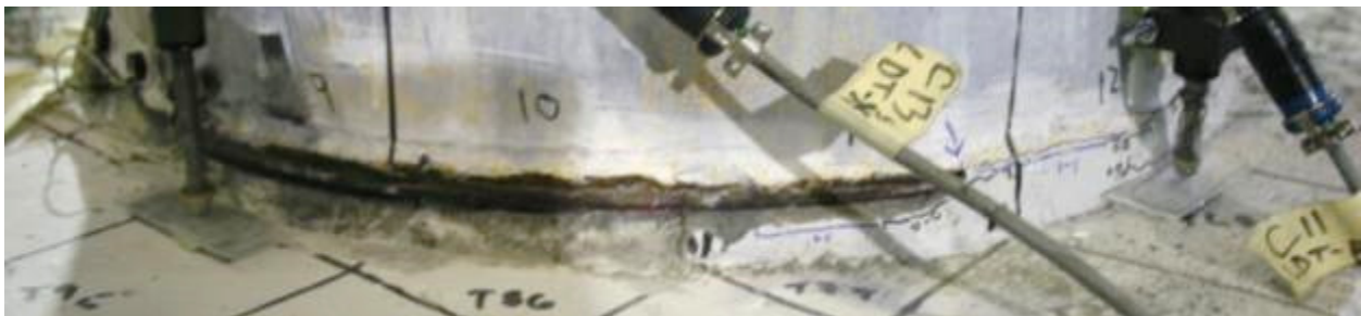
Figure 4.14 Southeast side of grout pad after test completion. The pad nearer the center of the connection remained largely intact.
