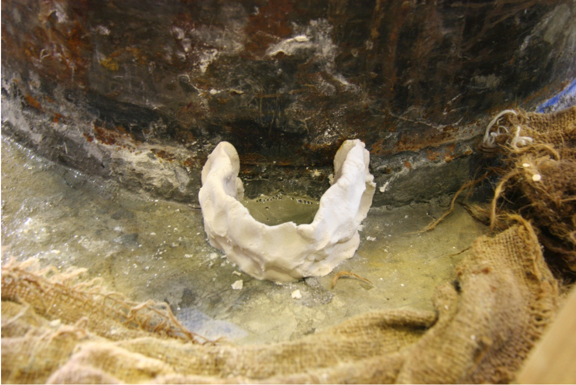
Figure 2.30 Pumped grout seeping from a bleed vent in the grout pad (excess grout was allowed to stiffen, and was then removed).
