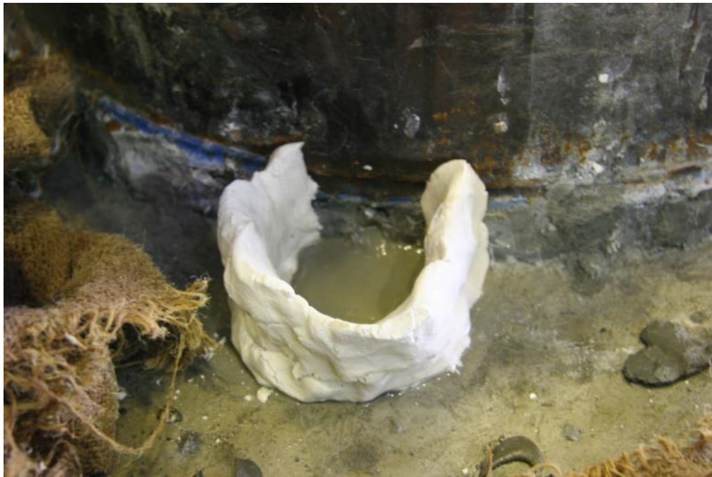
Figure D.18 Grout was pumped into ducts until it flowed out of vents left in pad, which then filled temporary reservoirs formed on top of the cap beam.
