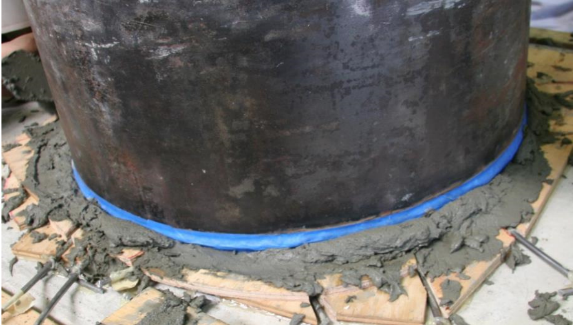
Figure D.15 Column was dropped onto fresh grout, and material was allowed to squeeze out from gap.
