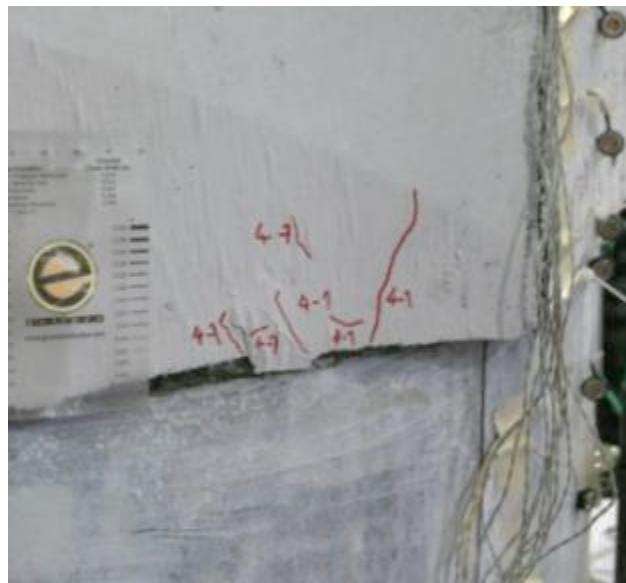
Figure 4.5 Minor surface flaking observed at the top of the steel tube.
