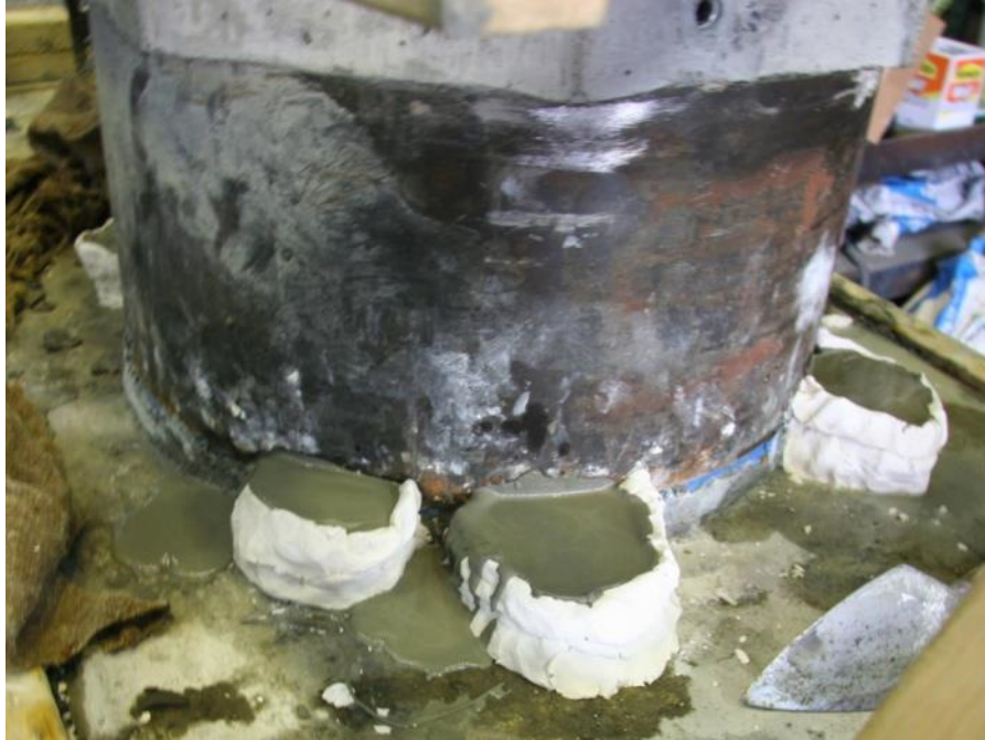
Figure D.19 Grout was pumped into ducts until reservoirs outside of vents were filled. This overflowing grout was allowed to setup and was then removed.
