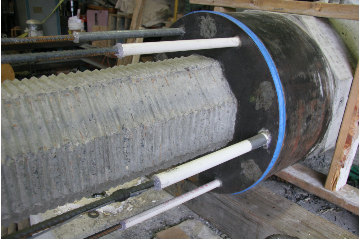
Figure 2.9 Debonding of protruding No. 4 bars. The PVC sheathed, north bars are on the right side of the photograph.
