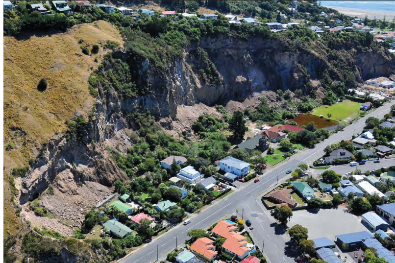
Figure 1.3: Rock and debris falls on 50m high cliff behind houses in Sumner, New Zealand [photo credit: GNS Science]
