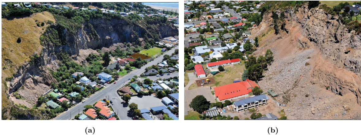
Figure 4.1: Cliff collapse at Richmond Hill (a) and Redcliffs (b) sites after the February 22, 2011 earthquake.[photo credit:GNS Science]
