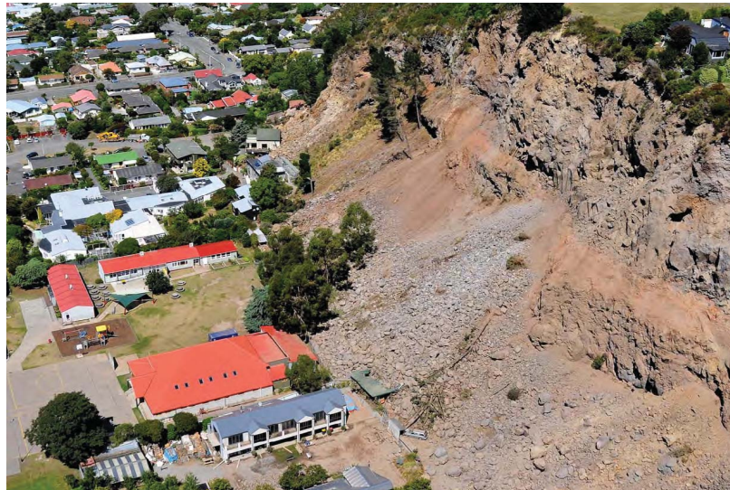
Figure 1.4: Large rock and debris falls on the 60m high cliff face behind Redcliffs School in Redcliffs, New Zealand [photo credit: GNS Science]
