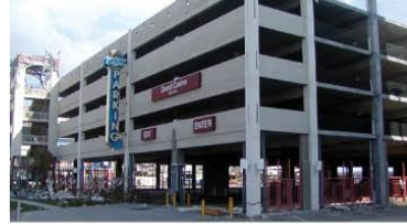
A reinforced concrete parking garage in Biloxi, Mississippi after Hurricane Katrina. Source: Guidelines For Design Of Structures For Vertical Evacuation From Tsunamis.
