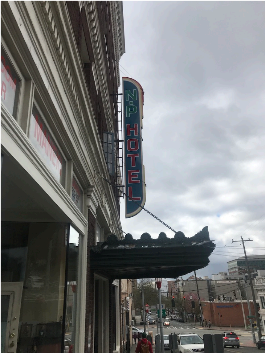
Figure 13: Neon NP Hotel sign and metal canopy on western façade (Source: Rachel Vickers, 2019)
