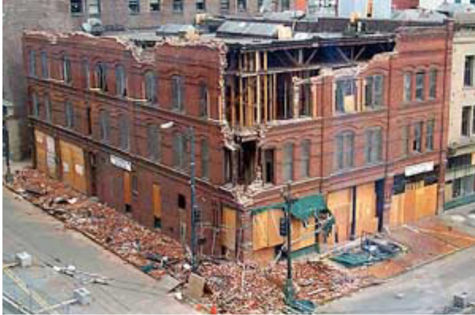
Figure 2: Cadillac Hotel damage from 2001 Nisqually earthquake (Source: Komo4 News, 2003)
