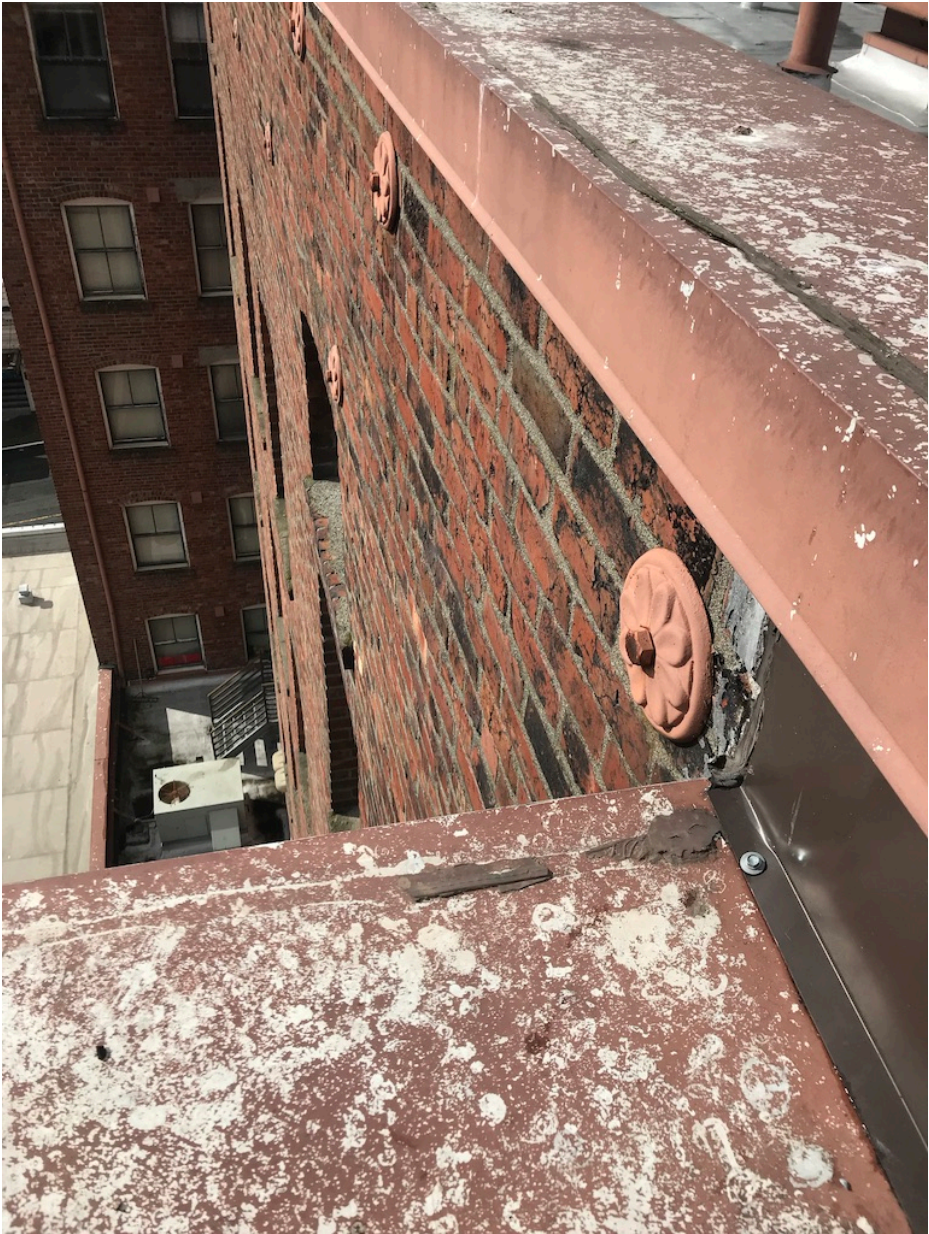
Figure 14: NP Hotel parapet bracing. Anchor bolts should match alignment and style of these bolts (Source: Rachel Vickers, 2019)
