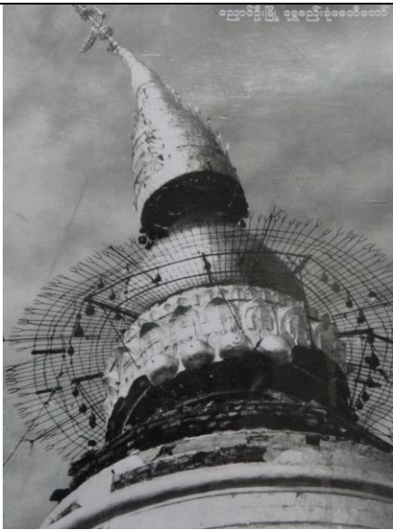
Figure 4.26 Bosses portion and the Hti were damaged in 1975 earthquake. (Provided by Shweziogn Gopaga)
