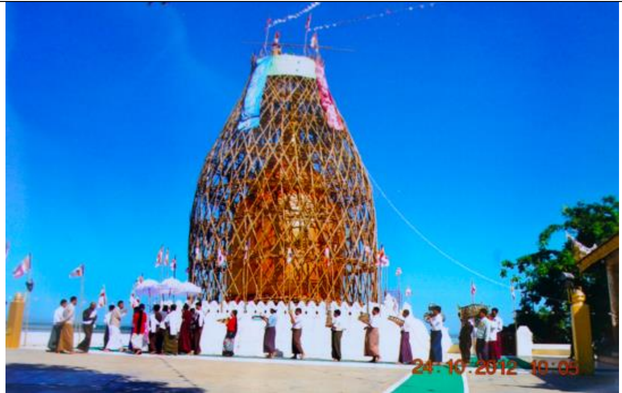
Figure 4.49. Before regilding and repairing the Hti, there's a ceremony after all part of the Hti had been unloaded. People would carry each portion to walk around the Bupaya pagoda for blessing later works in 2012.
