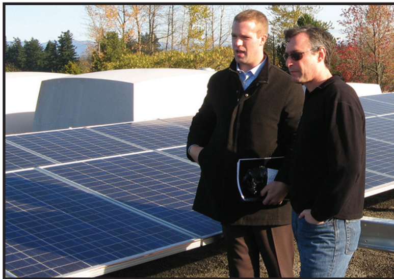
SunEdison program manager Jeremy Barnett (left) walks Multnomah County Commissioner Jeff Cogen through a photovoltaic array installed on the roof of the Yeon maintenance building. Because of the way the deal is structured, the $7 million-plus project is not subject to requirement to pay the prevailing wage. Photo courtesy of Multnomah County Commission
