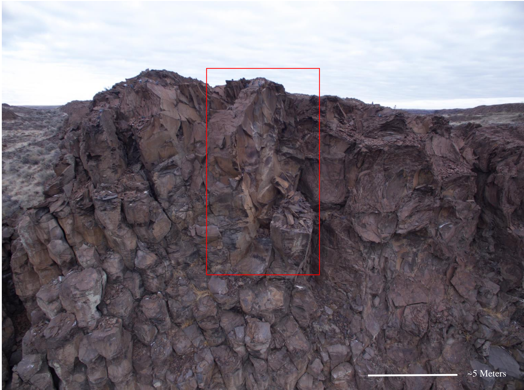
Close up image of detachment zone. The location from which the rock fall originated is outlined in red. Lighter colored surfaces are present showing where fresh fracture surfaces have been exposed. Some loose fractured rock material remains on the cliff face.
