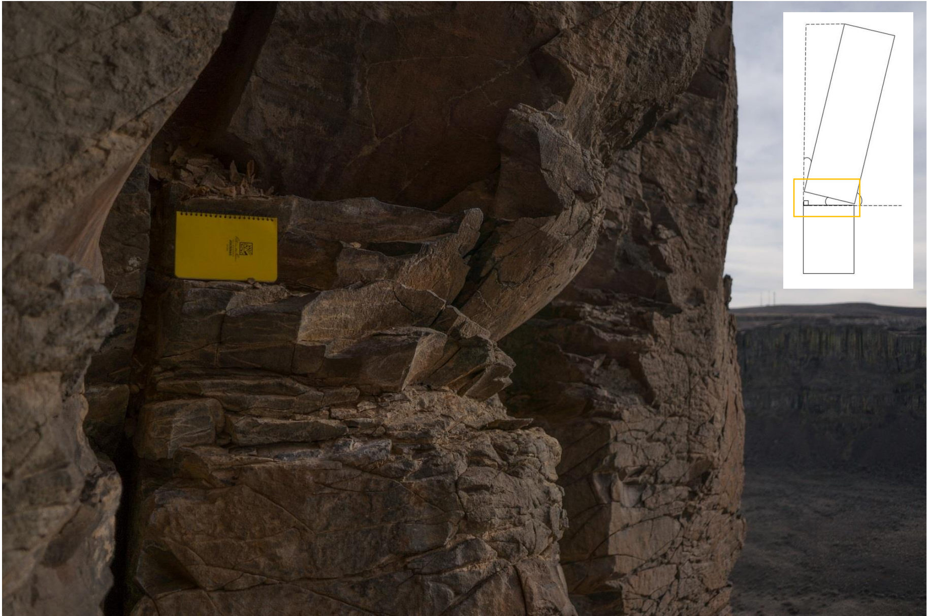
Figure 8: Platy Zone. Adjacent to the notebook is the low RMR zone. This particular column has already failed and only the lower 9 meters of the column remain. The remaining section of this column is supported by the neighboring intact column. The yellow notebook shown is 6 inches across, from left to right.
