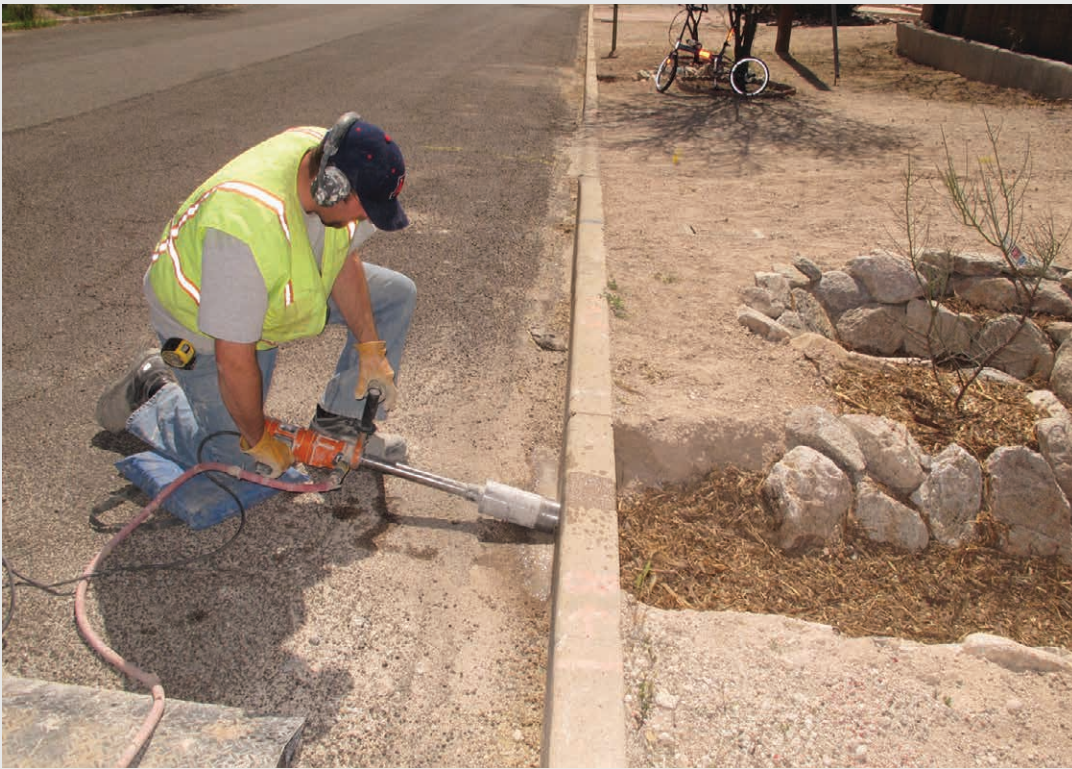
Figure 7.4: creating a curb cut in an existing curb using a hole saw (73)
