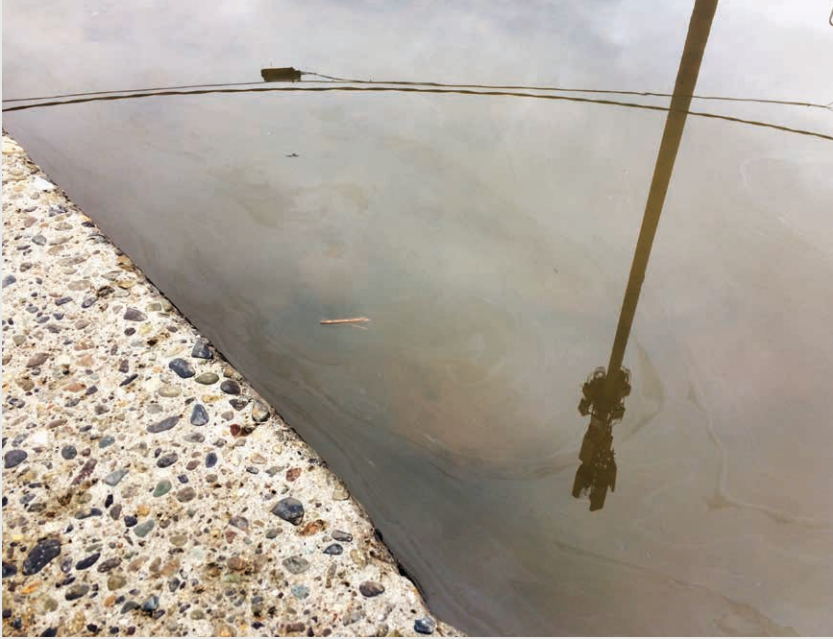
Figure 5.10: standing water with visible contamination
