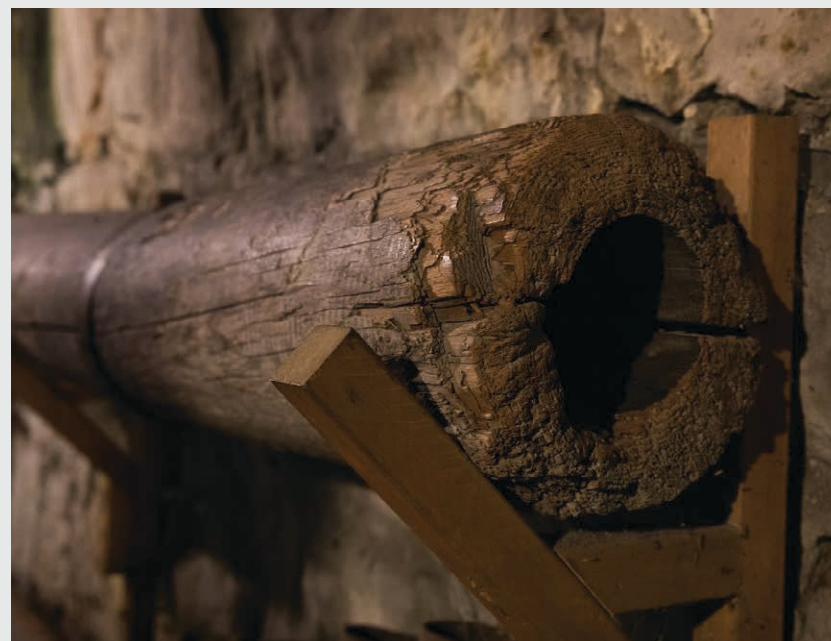
Figure 2.1: A wood stave pipe used to carry Seattle's water in the early 1900s (1)
