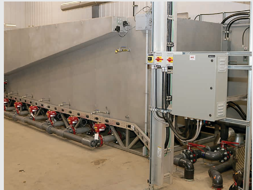
Figure 8.4: electroflocculation treatment infrastructure in Unity, SK (82)
