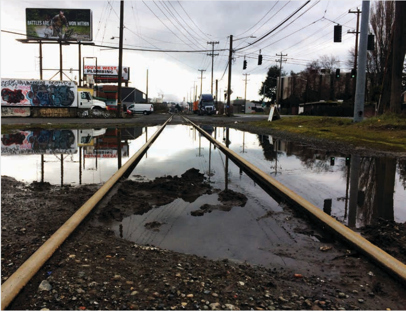
Figure 5.9: standing water on the railroad tracks near the Duwamish River
