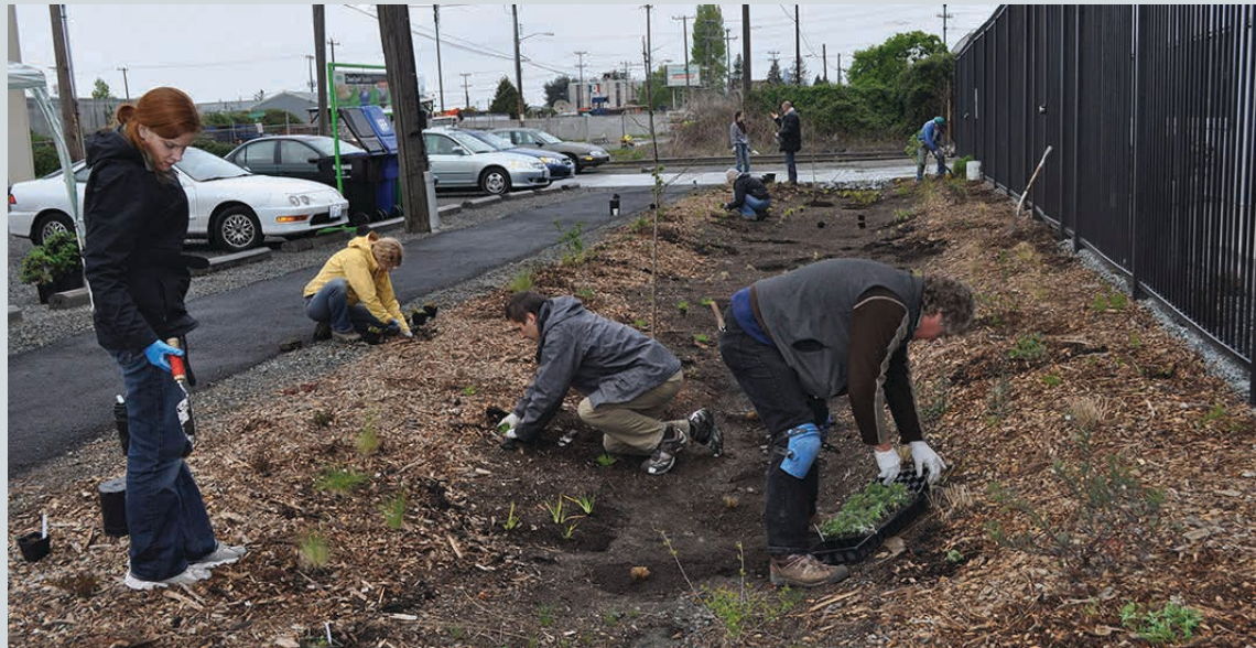
Figure 7.16: The Markey Machinery swales during planting by volunteers in 2010. Photo by Carl Simon (79)
