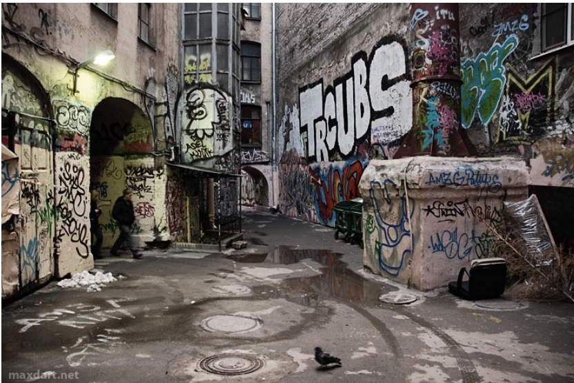
Fig. 6: Deteriorated courtyard with graffiti
