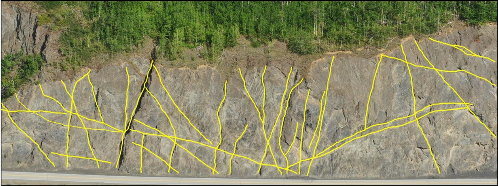
Figure 2.14 Long Lake (MP 71), Alaska, west section: major discontinuities (yellow) in mudstone.
