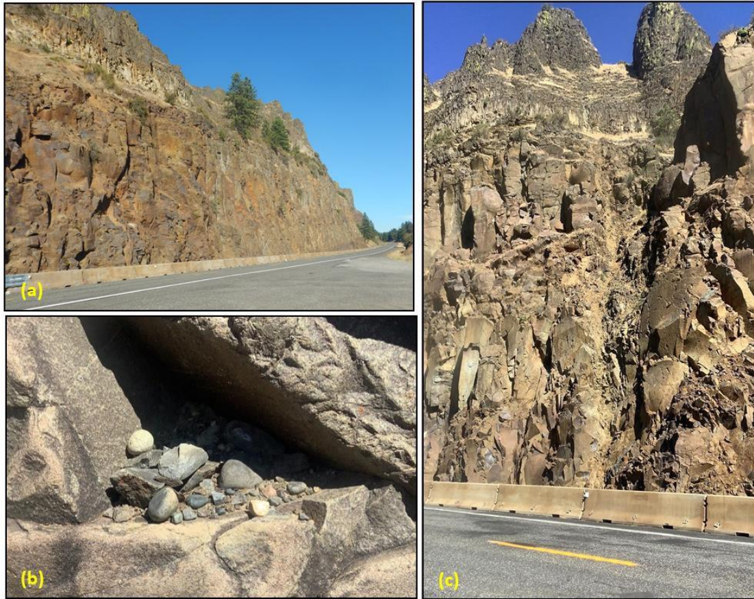
Figure 2.3 Views of the Hewett Lake (SR 14) research site: (a) view to the east along the highway; (b) example of the interpreted Missoula flood deposits nestled under an overhanging block; (c) example of a high-angle fault.
