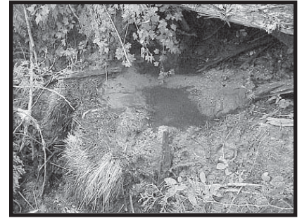
Filled sediment trap that is no longer serving its function. Flow is able to go around the trap unmitigated.
