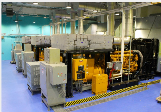
Image 72: Backup Generators. Located in a floodproof facility and are elevated off the ground (Johns Hopkins Medicine 2016).
