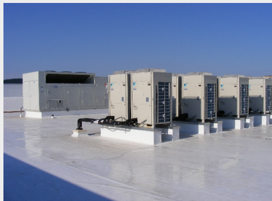
Image 75: Rooftop Equipment. Mechanical equipment is located on the roof. The higher elevation reduces its exposure to flooding (Fidelity Engineering Corporation 2013).
