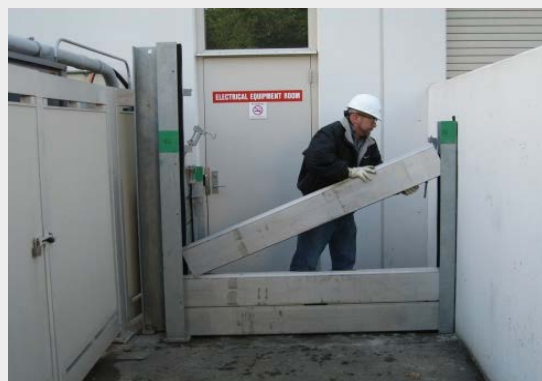
Image 73: Temporary Flood Barrier. A worker is installing a flood barrier to protect an electrical room in anticipation of a storm (Flood Control America 2016).
