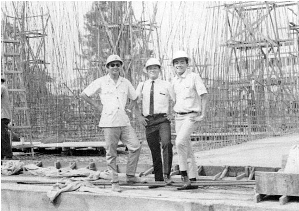
Figure 3-13 - The first Thai investor in high-rise building, Chokchai Bulakul, stood in the middle of the construction site of Chokchai International building (1969), Photograph, in Thailand Creative and Design Center, Keeping Up Modern Thailand (Bangkok: Thailand Creative and Design Center, 2008), 42.
