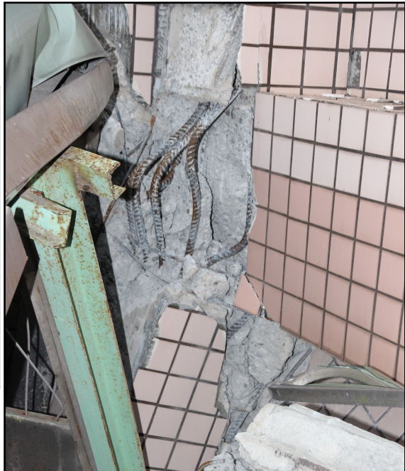
(d) Exposed and Buckled Rebar on Collapsed Side.
