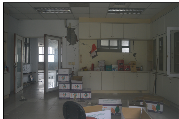
(f) Cracked Interior Wall
