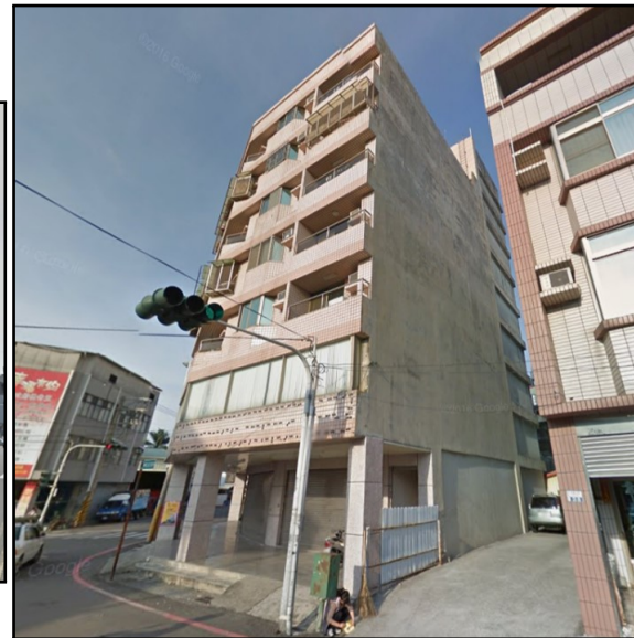
(b) RC Wall at South Face with View of Stair Core to the Far Right with Visible Beams
